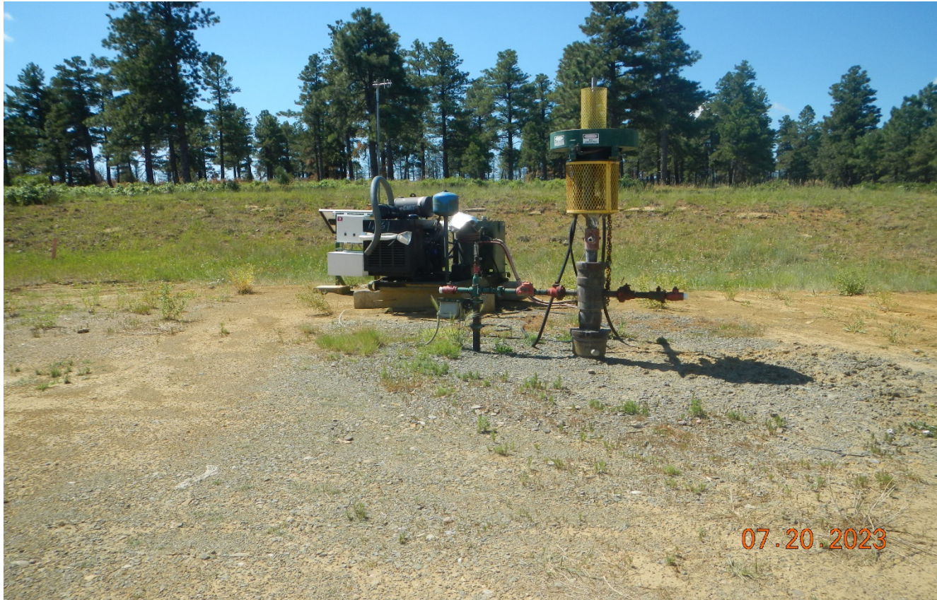
Photo 2. Facing toward the wellhead.
