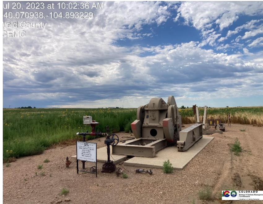
Pic 3 unused pumpjack on location needs to be removed.
