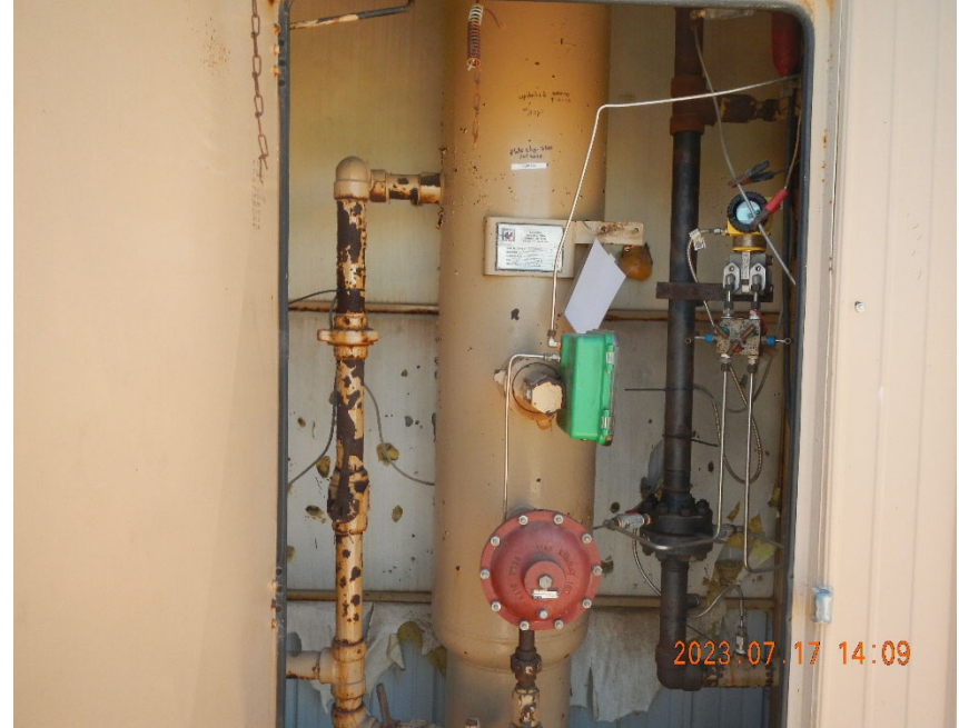
4. View of Vertical Separator and Digital Gas Meter Run inside Meter Shed.
