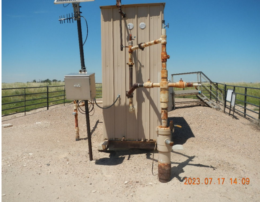
3. Wellhead and Gas Meter Shed.
