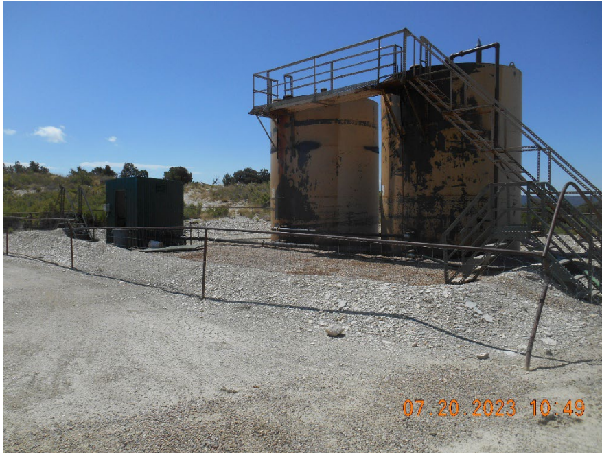
Tank battery and Pump housing
