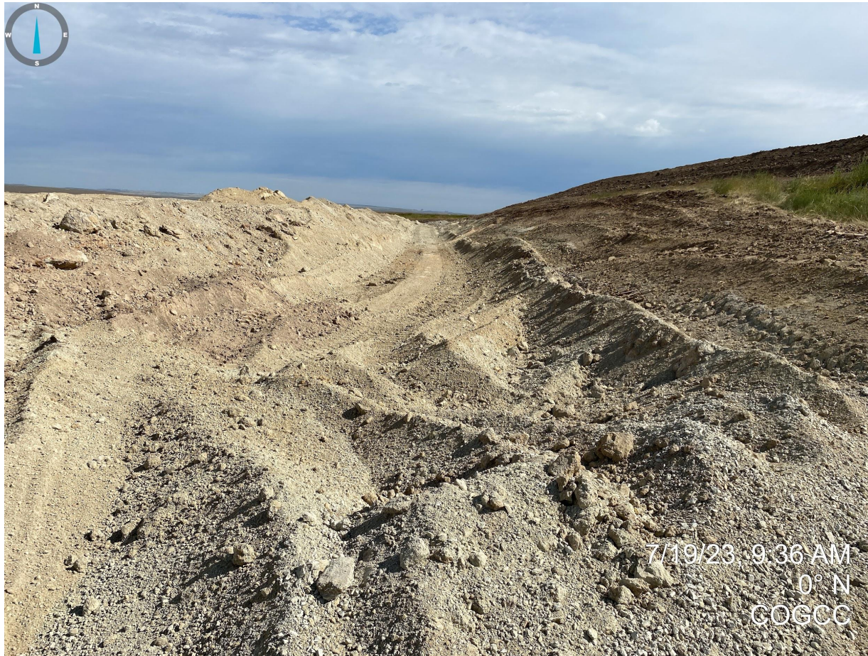
Photo 15. Facing north near the topsoil stockpile. Photo illustrates an apparent stormwater retention area still under construction.
