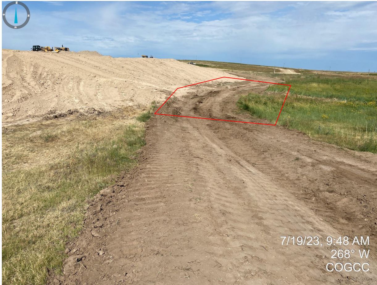
Photo 21. This area of the stormwater BMP (red outline) previously documented sediment transport due to unconsolidated materials. It appears the Operator has performed activities to repair/stabilize the unconsolidated soils.
