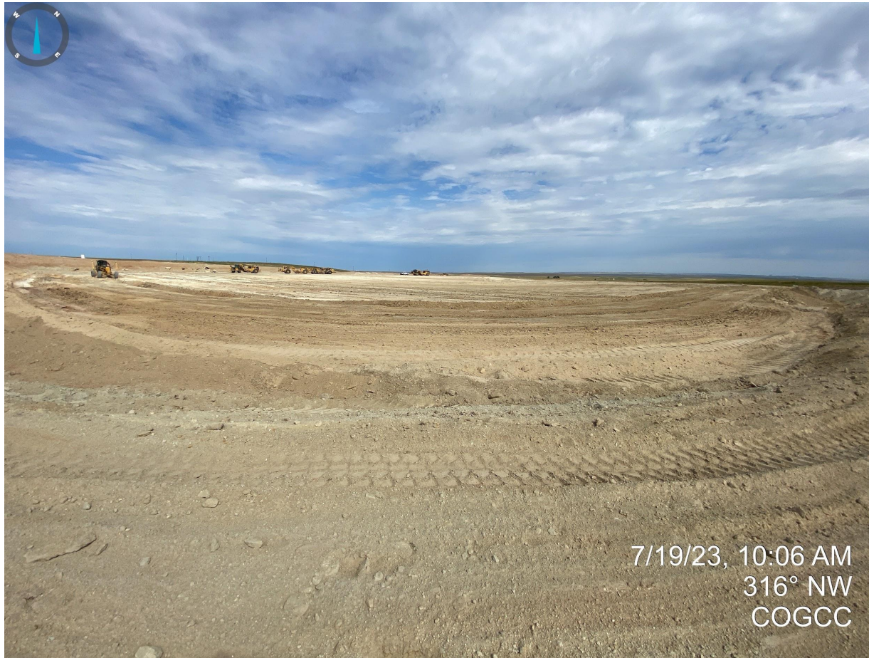
Photo 22. Taken from the southeast corner of the drilling pad area, facing northwest. Photo illustrates construction activities being performed. A follow up inspection will be performed at a later date to ensure compliance with ECMC Rules.
