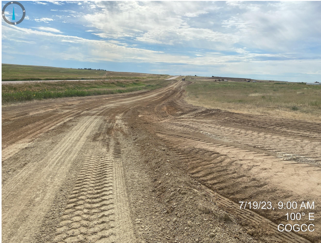
Photo 9. Facing east near the location's entrance. It appears topsoil has been salvaged and temporary BMPs (ditch and berm) have been installed alongside of the access road.
