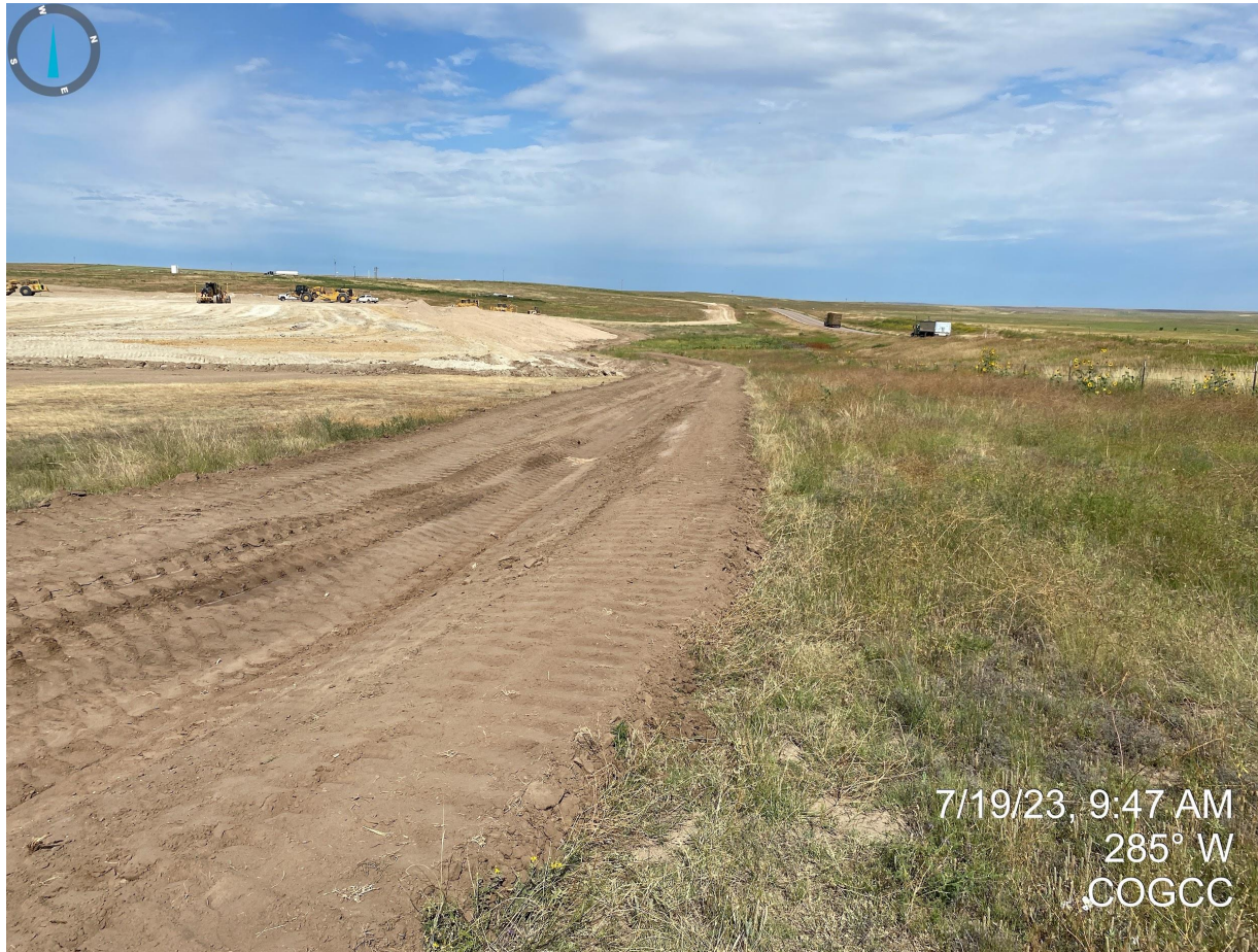
Photo 20. Facing west from the northeast corner of the disturbance area. Stormwater BMPs appear to have been improved/repared since the previous inspection.
