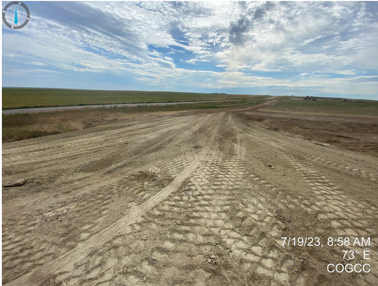
Photo 4. Taken from the location's current access road near the intersection of WCR 113 and HWY 14. No BMPs (e.g. vehicle track out pad) were installed at this junction. Proceeding photos illustrate vehicle track out onto HWY 14.
