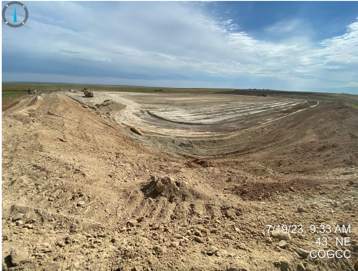
Photo 13. Taken from the southeast corner of the newly constructed drilling pad areas. Photo illustrates cut and fill slopes in foreground and production area in the background. Crews were onsite during this inspection and were actively performing dirt work to stabilize cut banks and fill areas.
