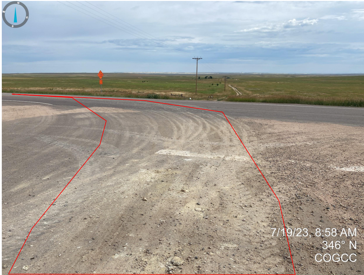
Photo 6. Vehicle track out pictured onto HWY 14 westbound.
