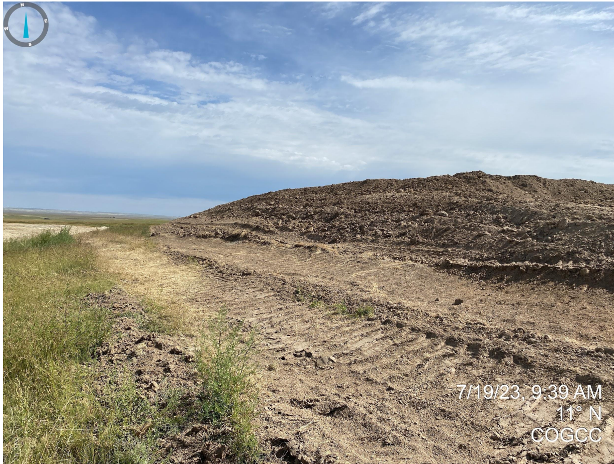
Photo 17. Taken from the southwest corner of the topsoil stockpile. It appears that topsoil has been separated and stored east of the disturbance area, in accordance with Rule 1002.b. However, the topsoil stockpile did not have any temporary BMPs (e.g. equipment tracking) to properly stabilize the soils from degradation due to wind and water erosion, etc. Additional BMPs are required to protect the topsoil stockpile on location and come into compliance with Rule 1002.c.
