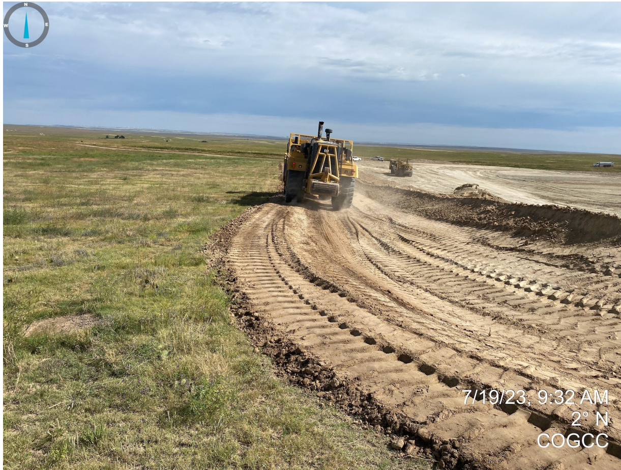
Photo 11. Taken from the southwest corner of the location. At the time of this inspection, crews were actively working to improve and/or maintain the perimeter stormwater BMPs. Vehicle wheel packing observed to mitigate unconsolidated material.
