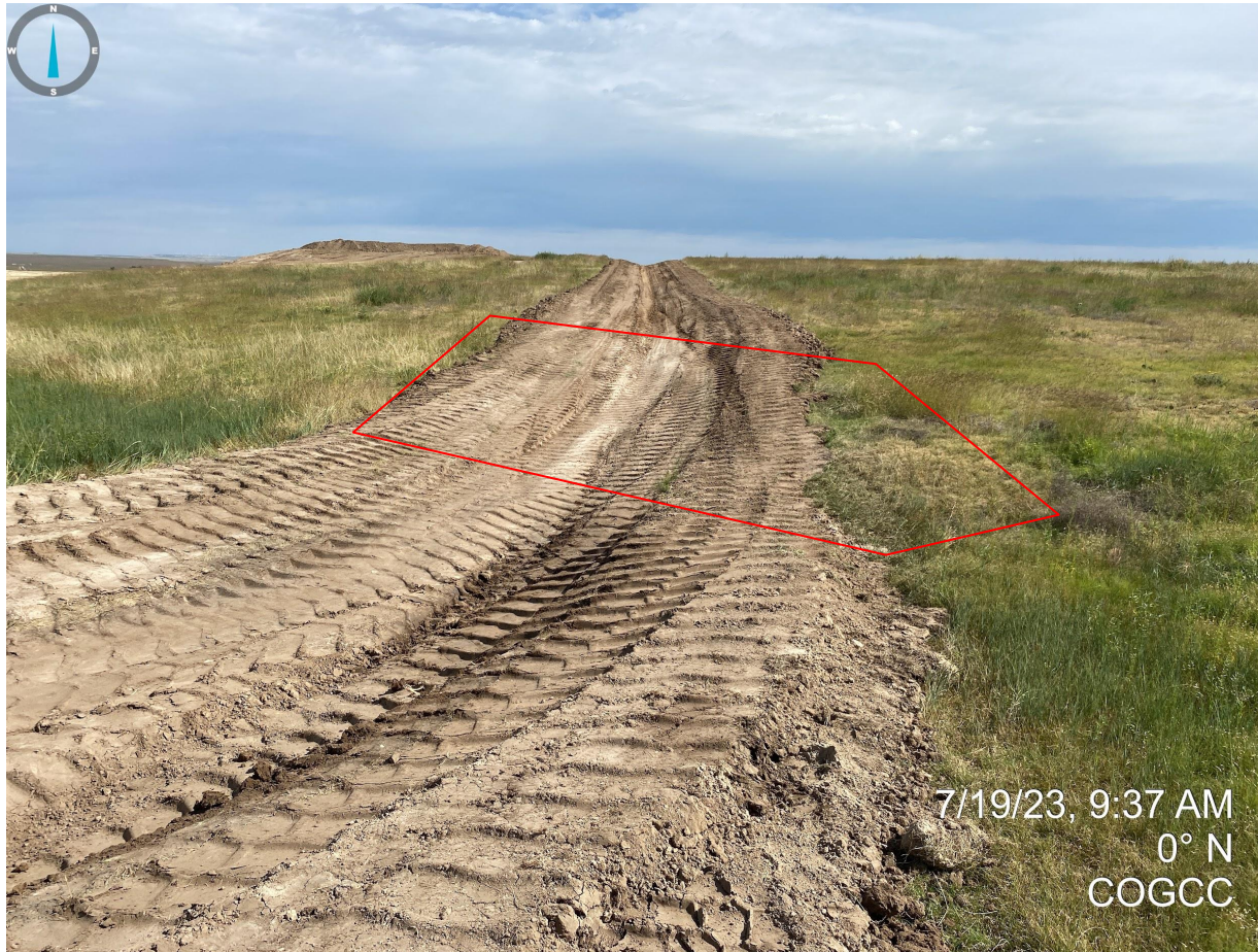
Photo 16. This area of the stormwater BMP (red outline) previously documented sediment transport due to unconsolidated materials. It appears the Operator has performed activities to repair/stabilize the unconsolidated soils.
