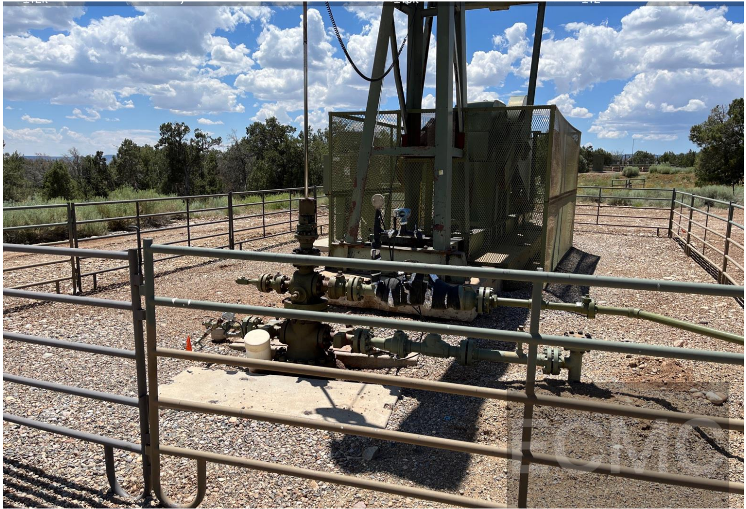
Photo #2. View of the wellhead assembly.
