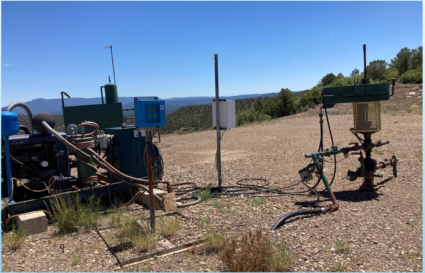
PHOTO 3: WELLHEAD AND EQUIPMENT
