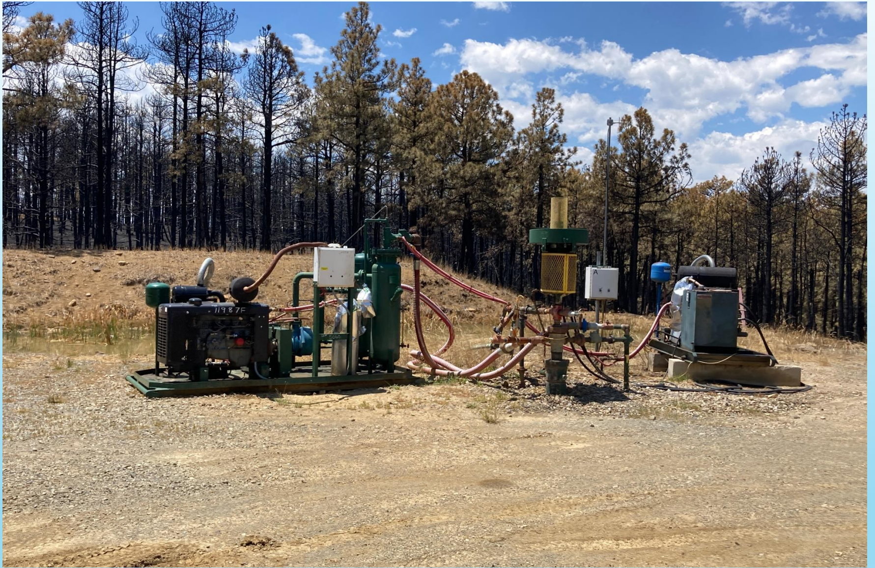
PHOTO 3: WELLHEAD AND EQUIPMENT
