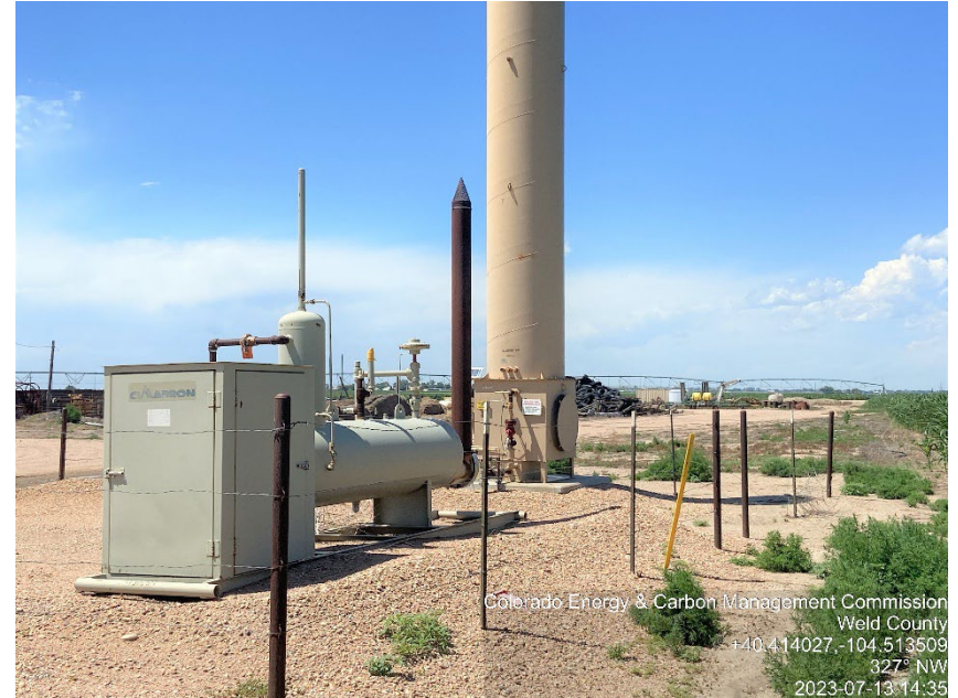
Photo #4 Trebor B 11-22 Battery site Inactive | Shut-down Separator(s), ECD(s)
