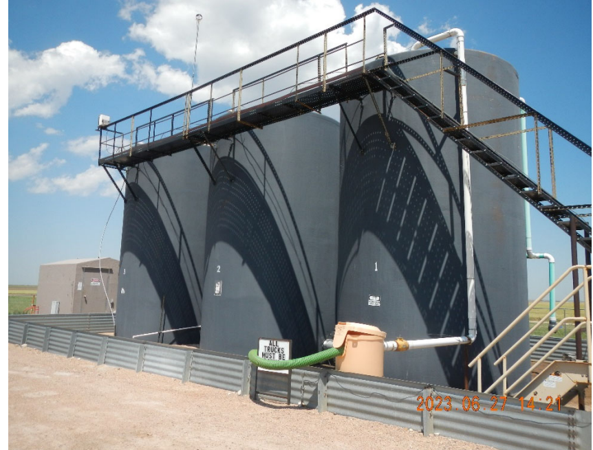
10. Back side view of tank battery.
