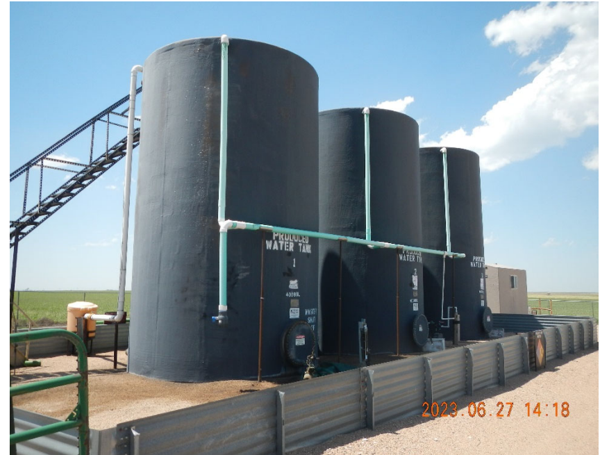
6. View of the three 400 BBL water tanks.
