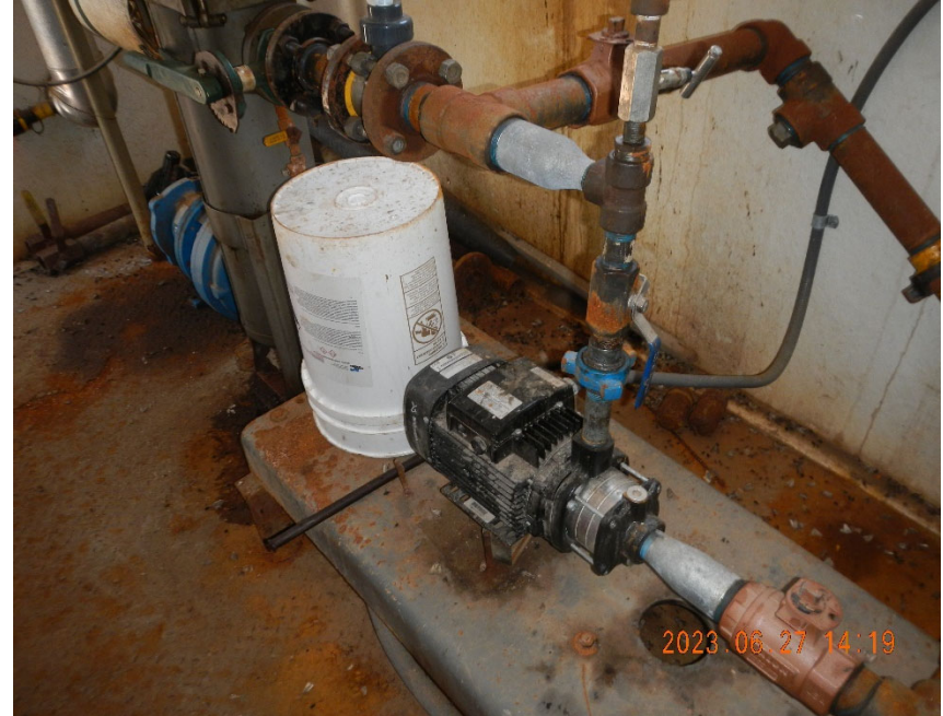
8. Pump inside injection building.
