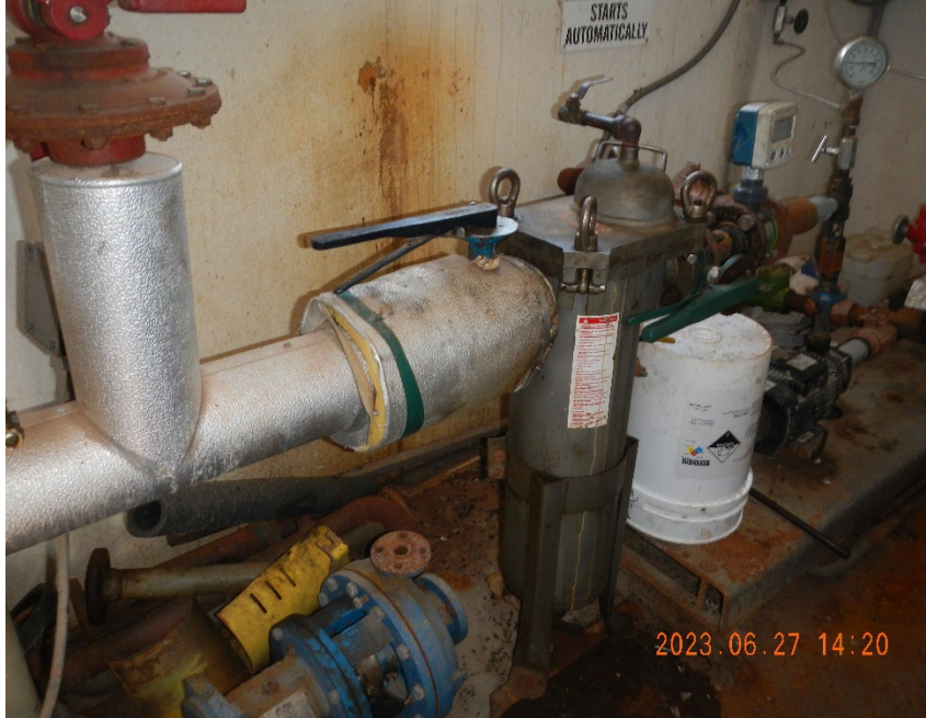
9. Water filter inside of injection building.
