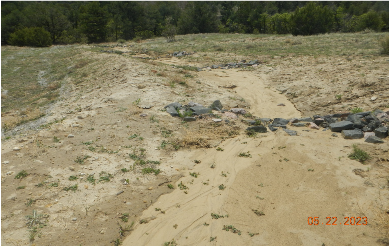
Photo 12. Facing south at the perimeter ditch. The check dams have filled in with sediment and need to be cleaned out.
