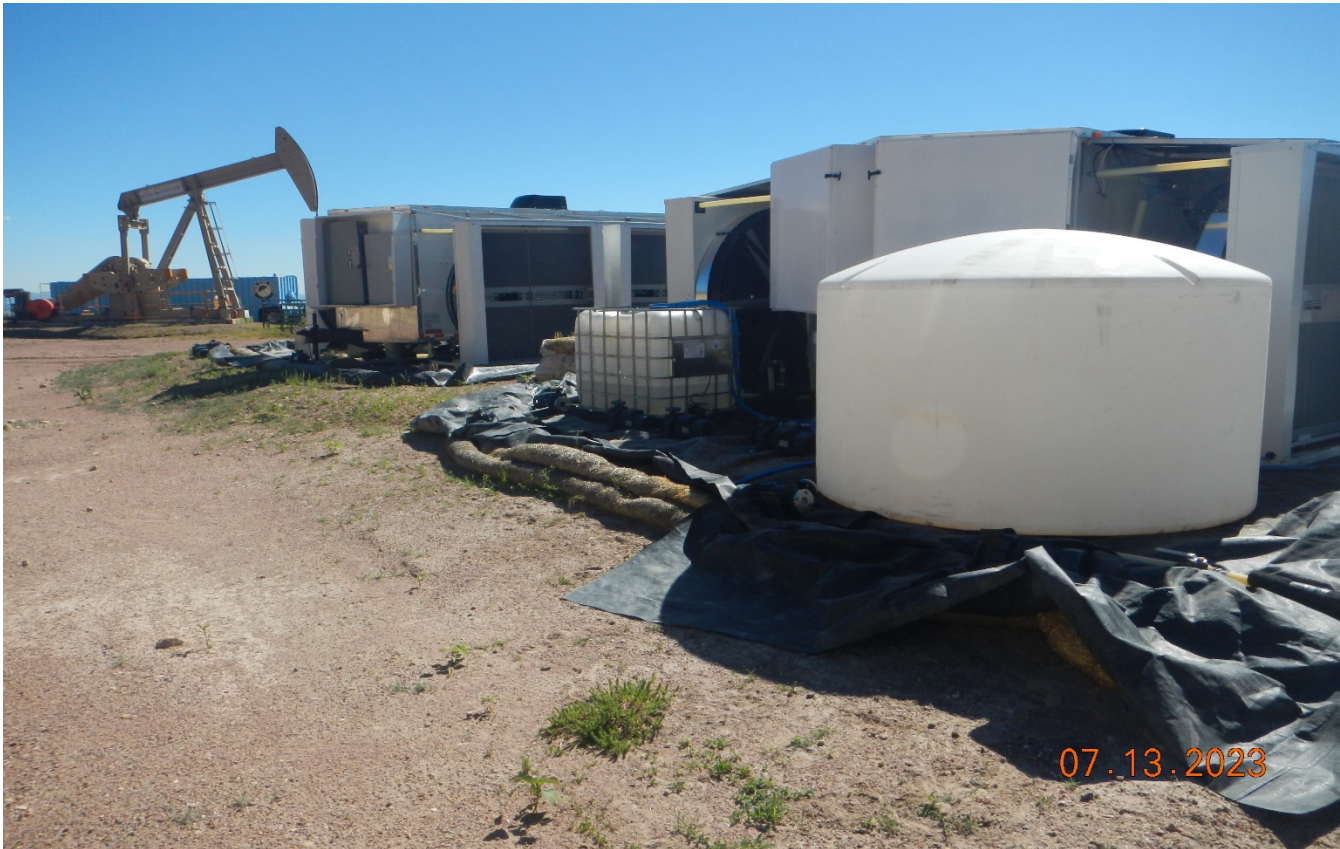
Photo 9. Northeast toward the bitcoin equipment. There are multiple tanks and secondary containment is not sufficient or maintained to contain a spill.
