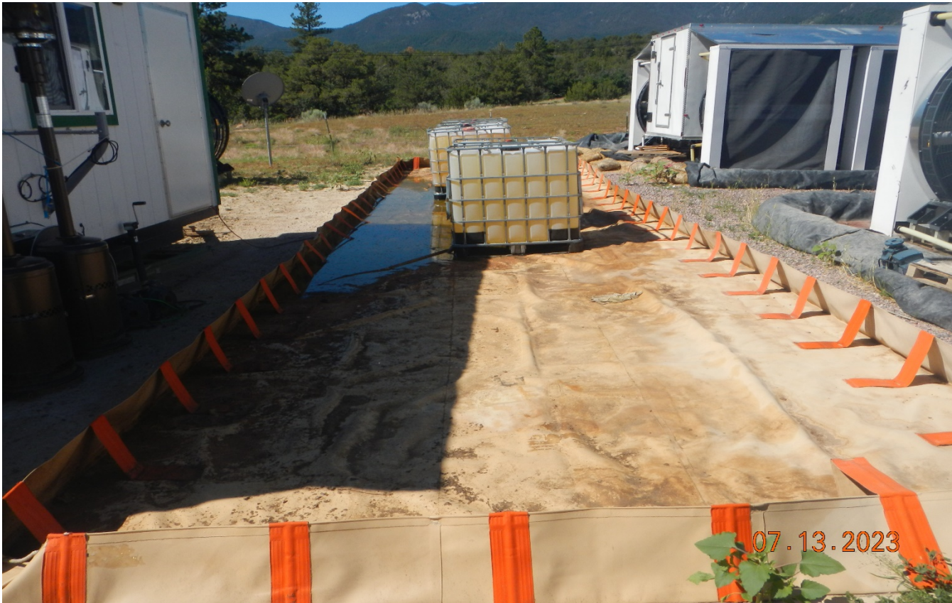
Photo 6. There is a portable secondary containment installed for the 2 chemical totes.
