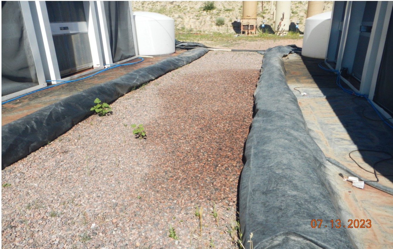
Photo 8. It appears in between the equipment there is darkened gravel from a possibly leak. Previous corrective action was not completed.
