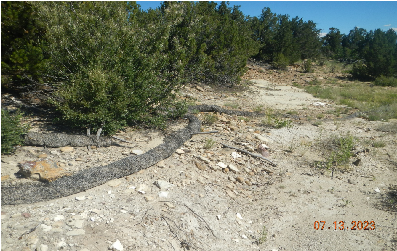
Photo 14 The wattles along the west perimeter of the location are degraded and need to be replaced or removed.
