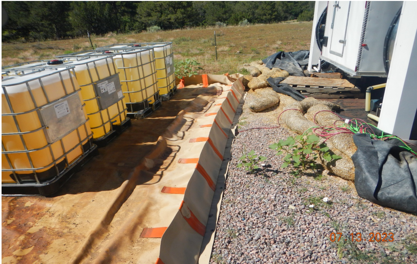
Photo 7. The plastic liner has become folded over needs to be repaired.
