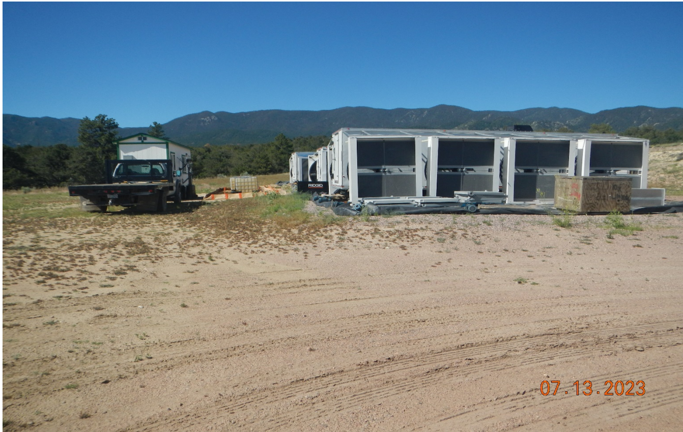
Photo 5. Facing southwest toward the bitcoin equipment which is not in operation.
