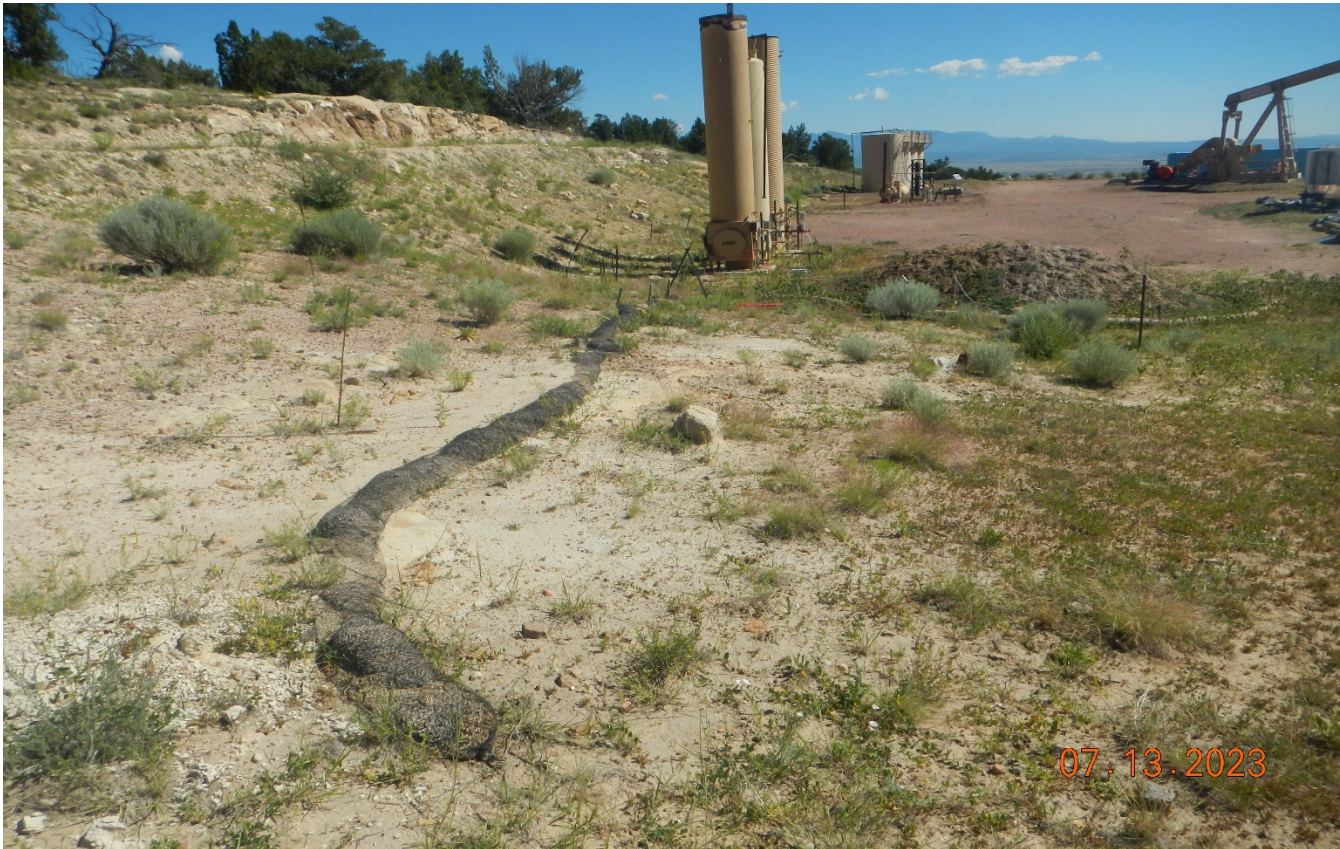
Photo 11. South side of the location facing northeast. The old wattles in this area need to be replaced or removed. Previous corrective action was not completed.
