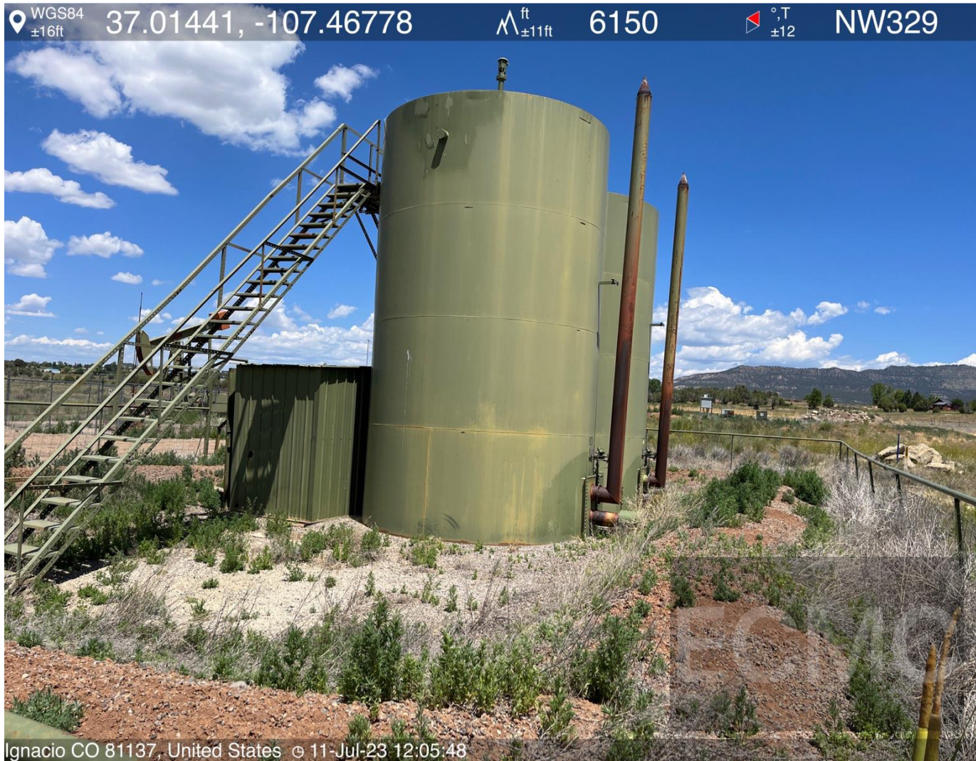
Photo #2. View of weeds growing on the tank battery containment berm.
