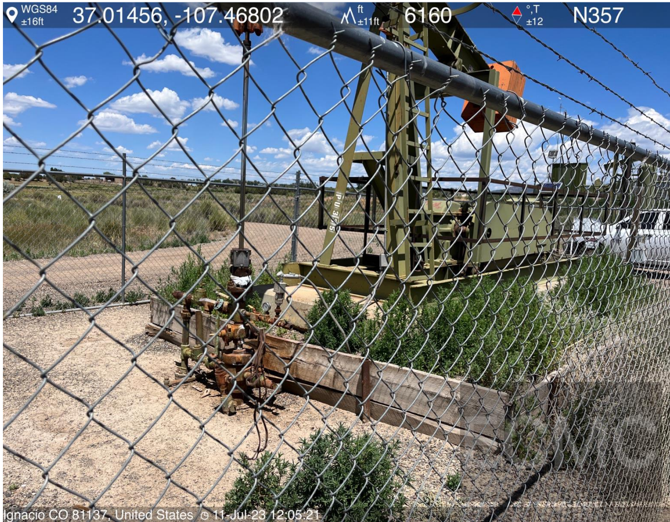
Photo #1. View of the wellhead assembly and weeds.
