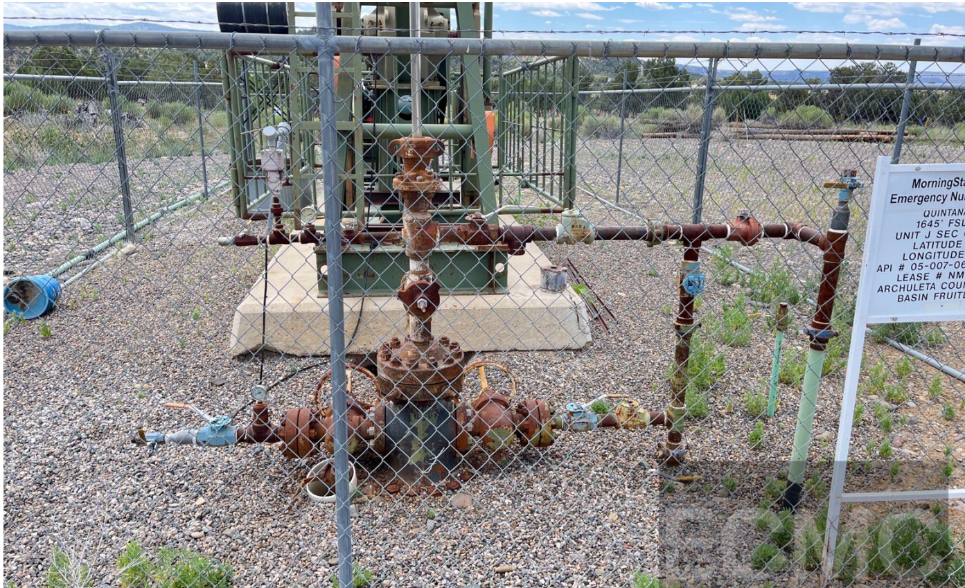
Photo #2. View of the wellhead assembly.
