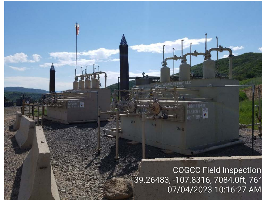
Photo #10 – Separators located at NE end of pad.
