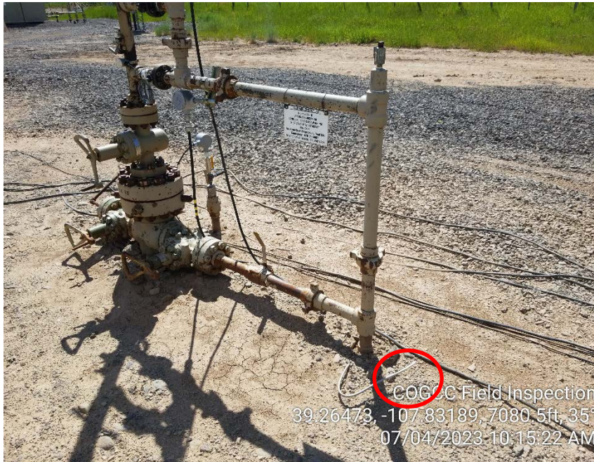
Photo #9 - Uncapped production pipe located at Nichols 24-10 wellhead.
