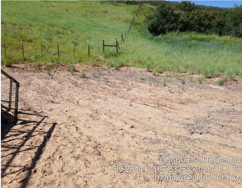
Photo #3 – Rutted area SW of tank battery.
