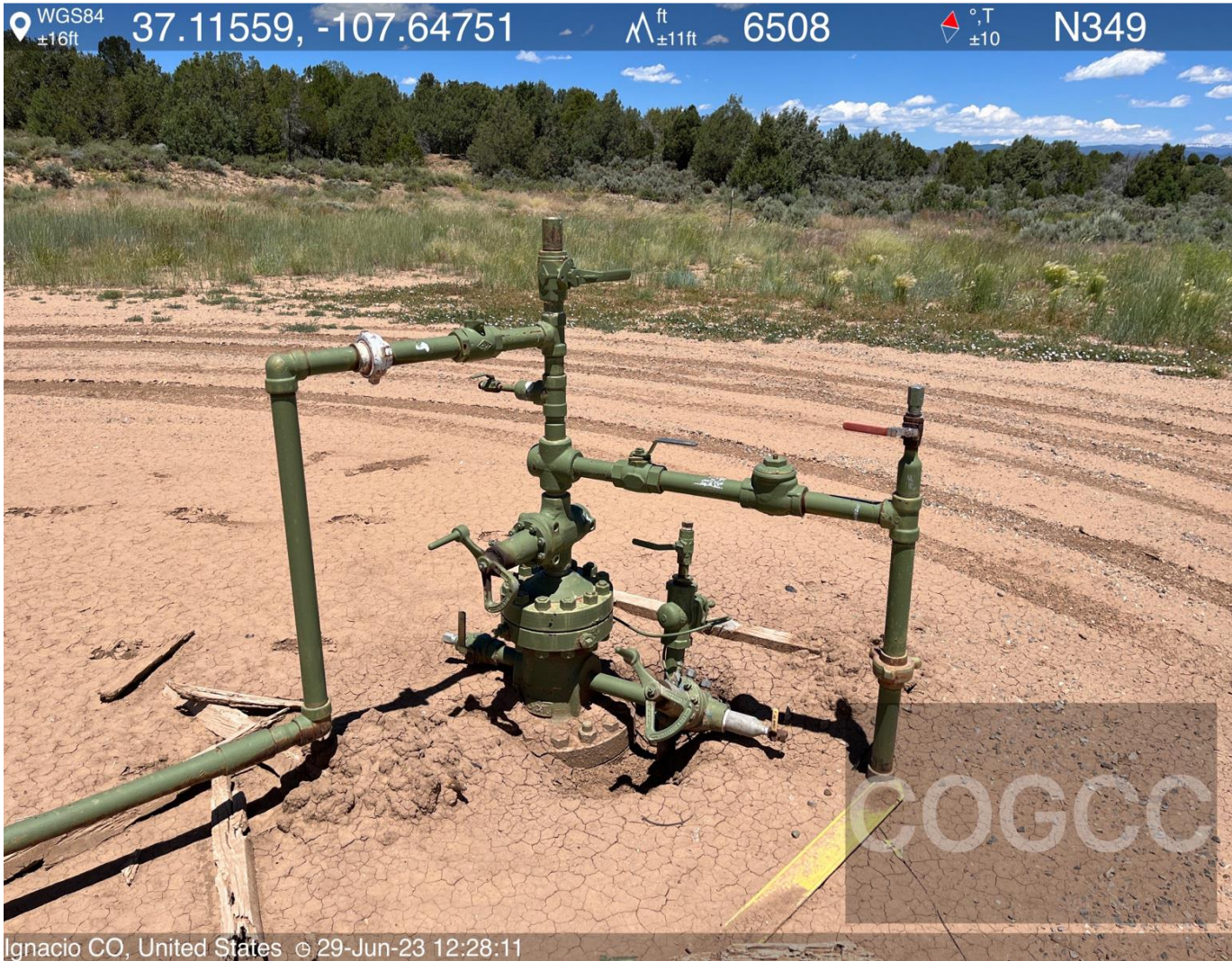
Photo #2 View of the wellhead assembly.
