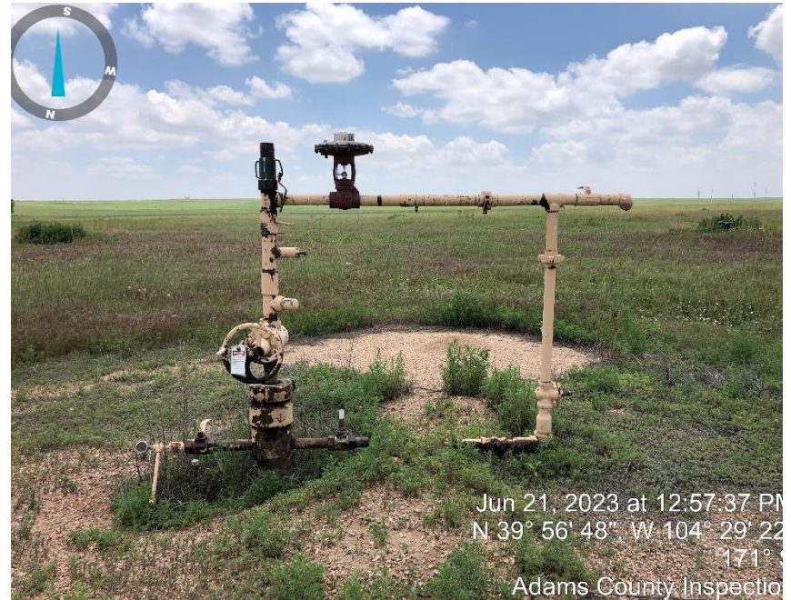
Photo# 4 Well head.
