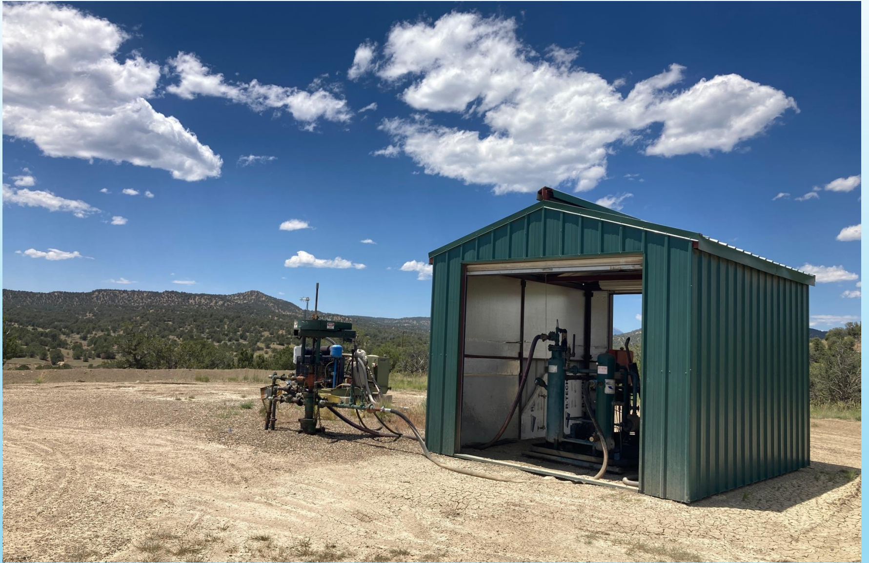
PHOTO 3: WELLHEAD AND EQUIPMENT
