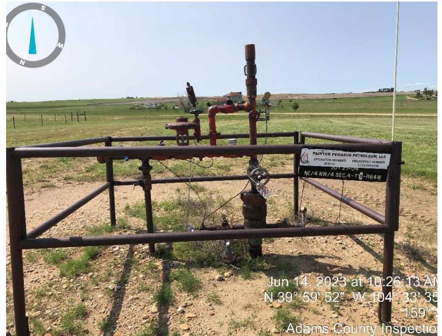
Photo# 4 Well head.
