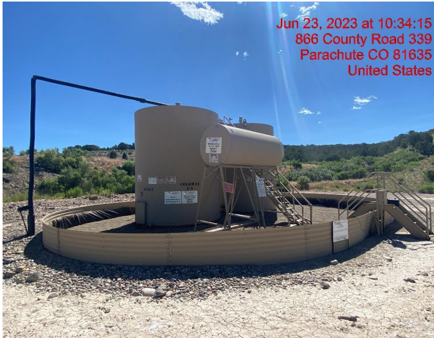
Tank Battery – Photo #04772
