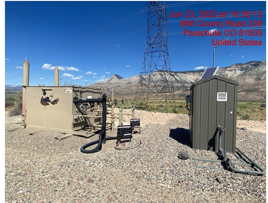
Separators/Gas Meter – Photo #04776
