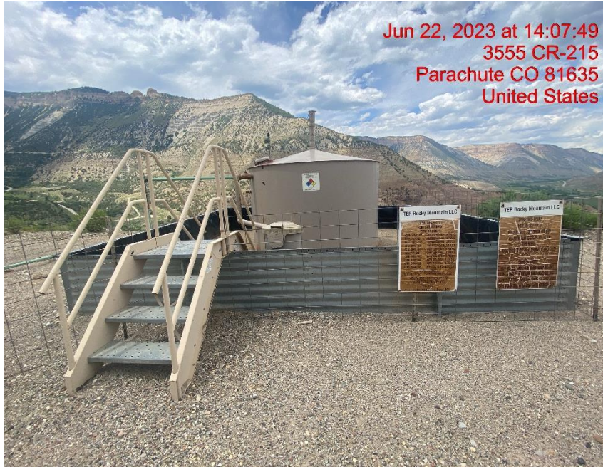
Tank Battery – Photo #04716
