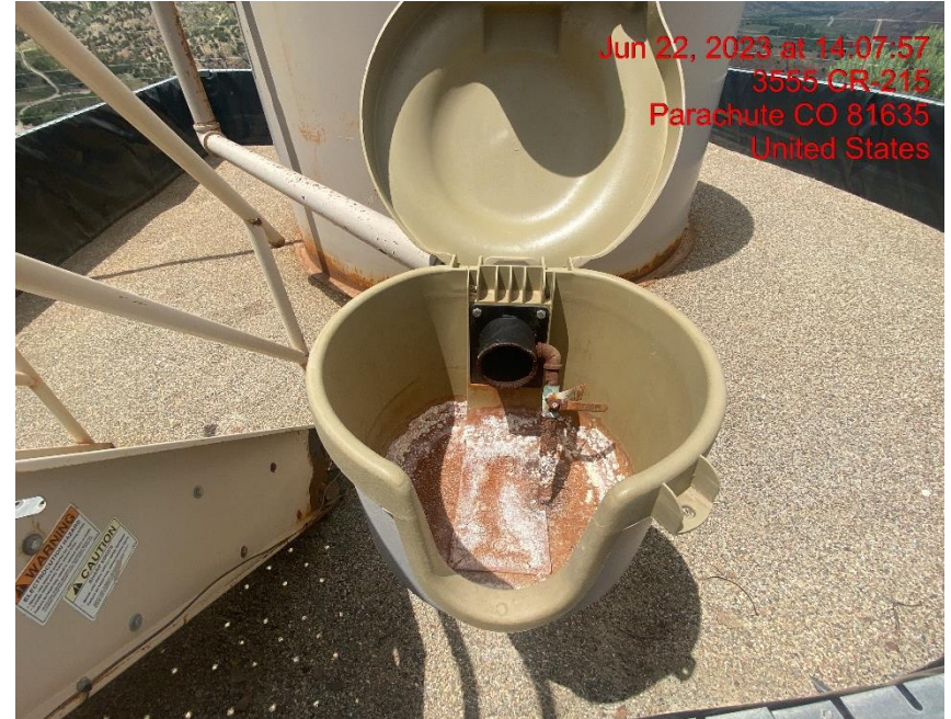
Open-Ended Load Line – Photo #04717
