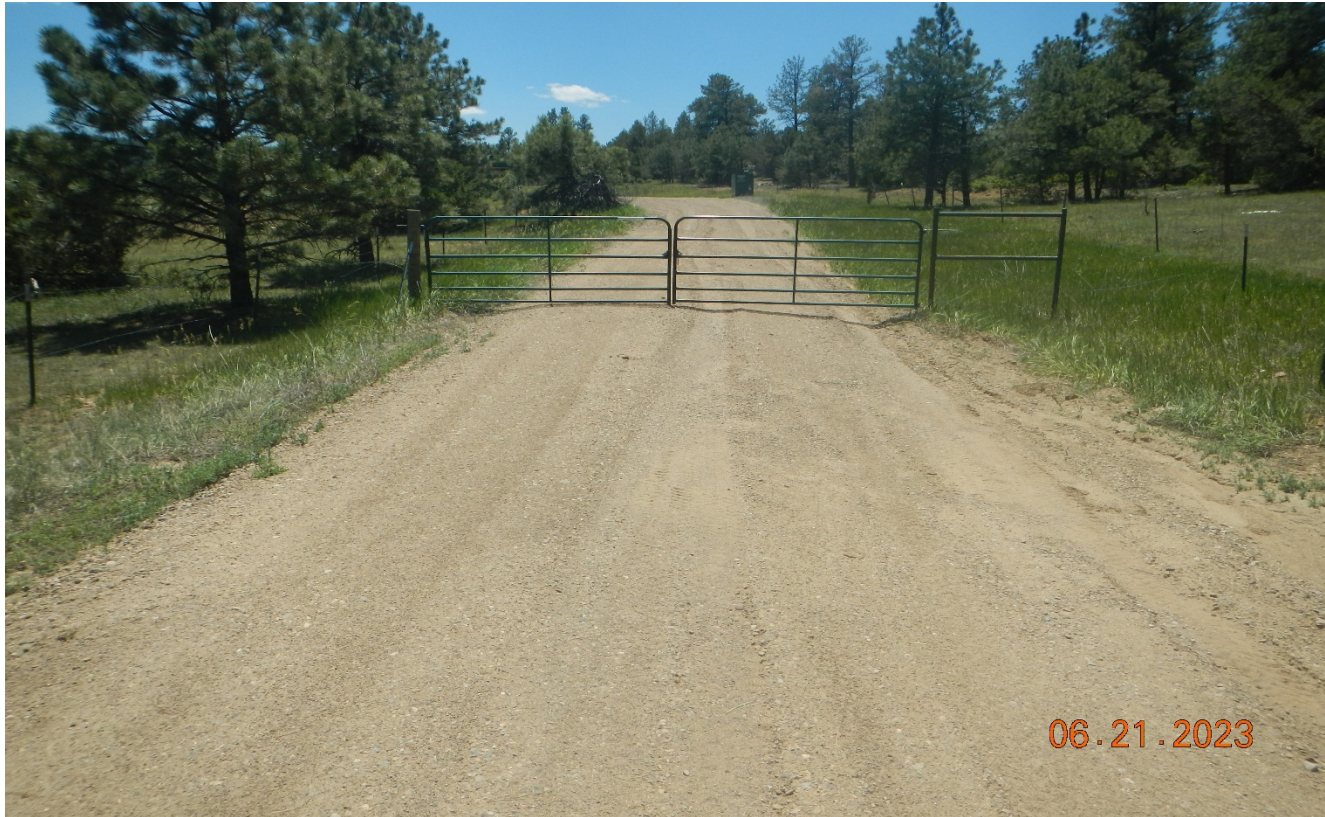
Photo 1. Facing south toward the access road which has been repaired and stabilized.
