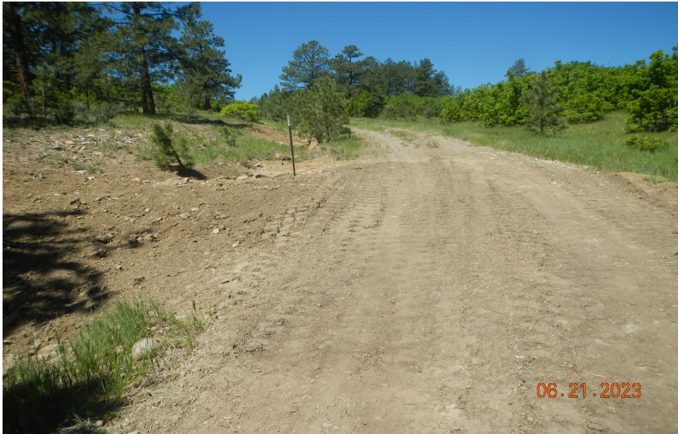
Photo 2. Further up the road the culvert has been repaired and is maintained.
