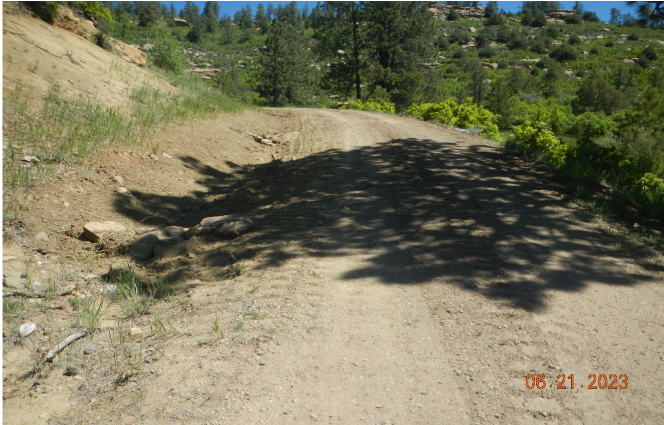
Photo 1. Facing north along the access road. The erosion along the road has been repaired and BMP's are maintained.
