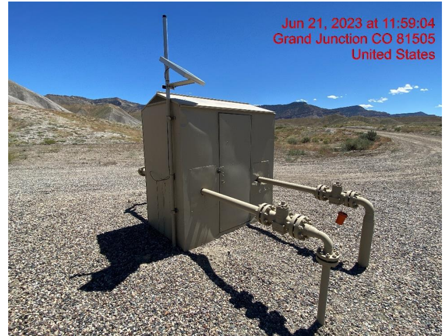
Gas Meter – Photo #04655
