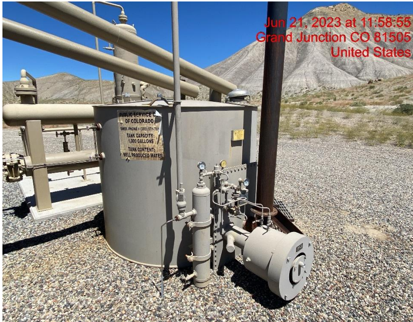
Produced Water Tank – Photo #04654
