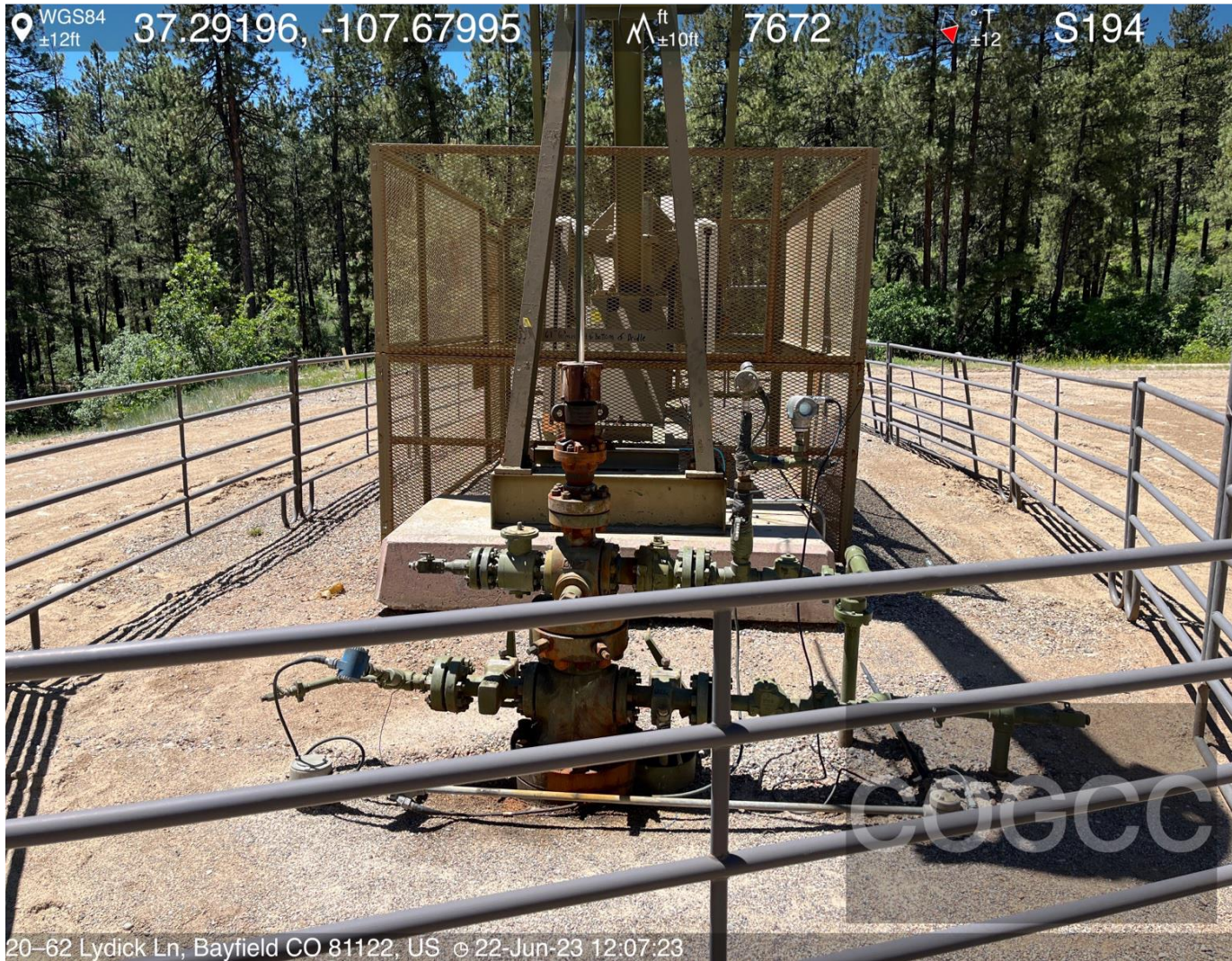
Photo #2 View of the wellhead assembly.
