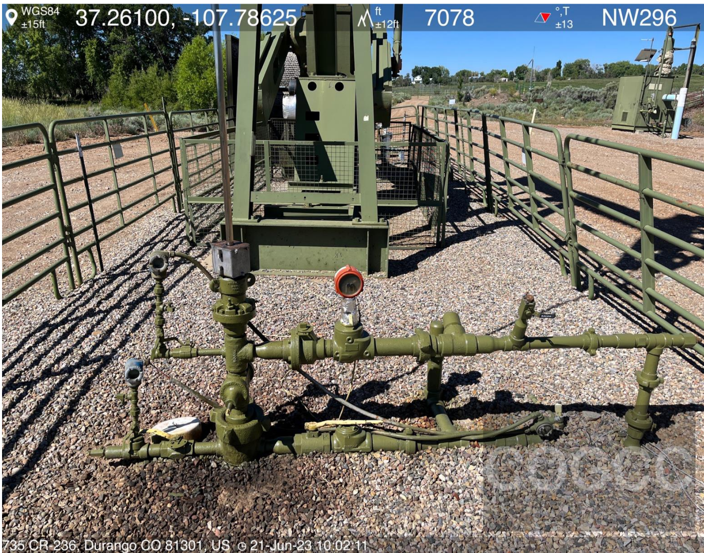
Photo #2 View of the wellhead assembly.
