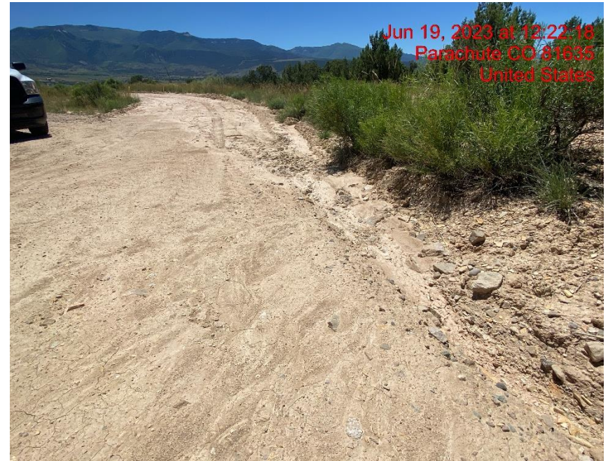
Access Road Ditch Full of Sediment/Needs Maintenance – Photo #04587
