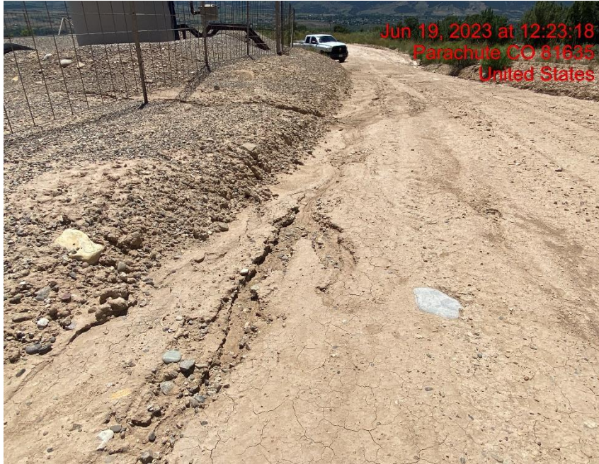
Rill Erosion on Access Road/Insufficient Vehicle Tracking BMPs at Location Entrance/Exit – Photo #04591
