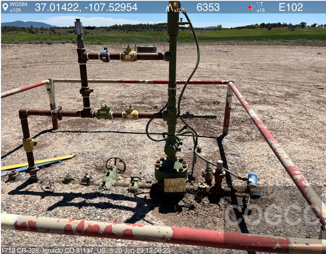
Photo #1 View of the #17-1 wellhead assembly.
