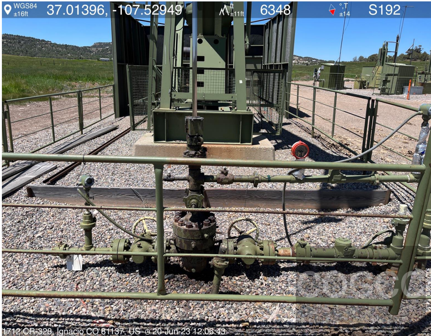
Photo #2 View of the #17-2 wellhead assembly.
