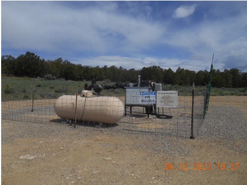
Injection wellhead & line heater
