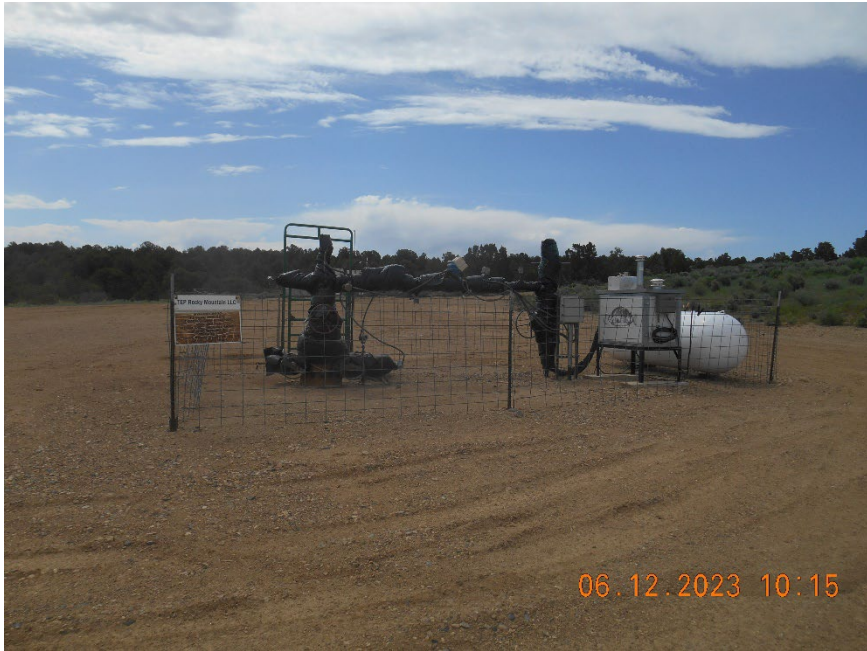
Injection wellhead & line heater
