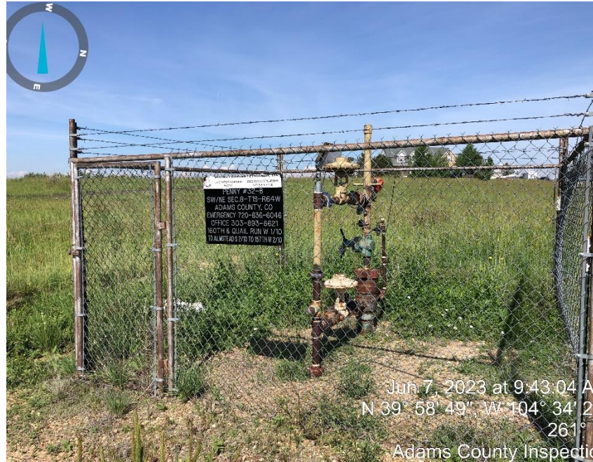
Photo# 1 Well head.
