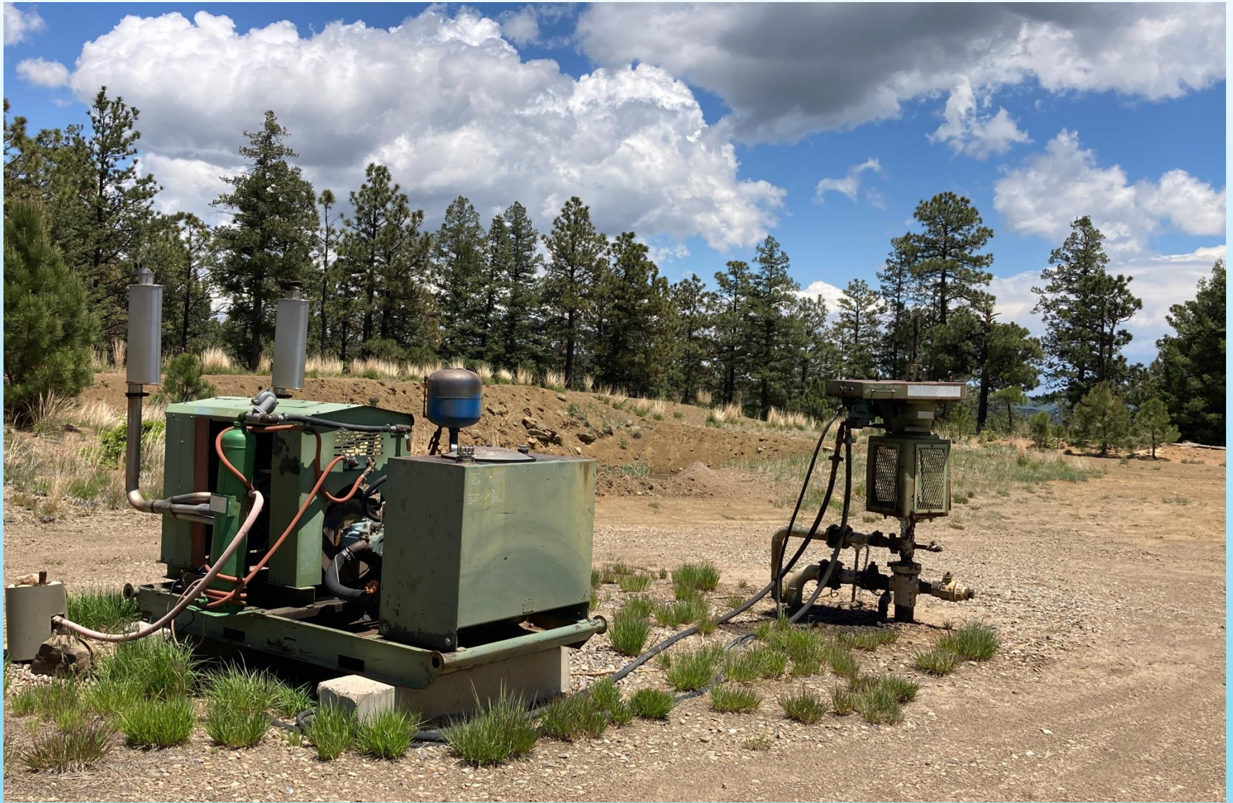
PHOTO 3: WELLHEAD AND EQUIPMENT
