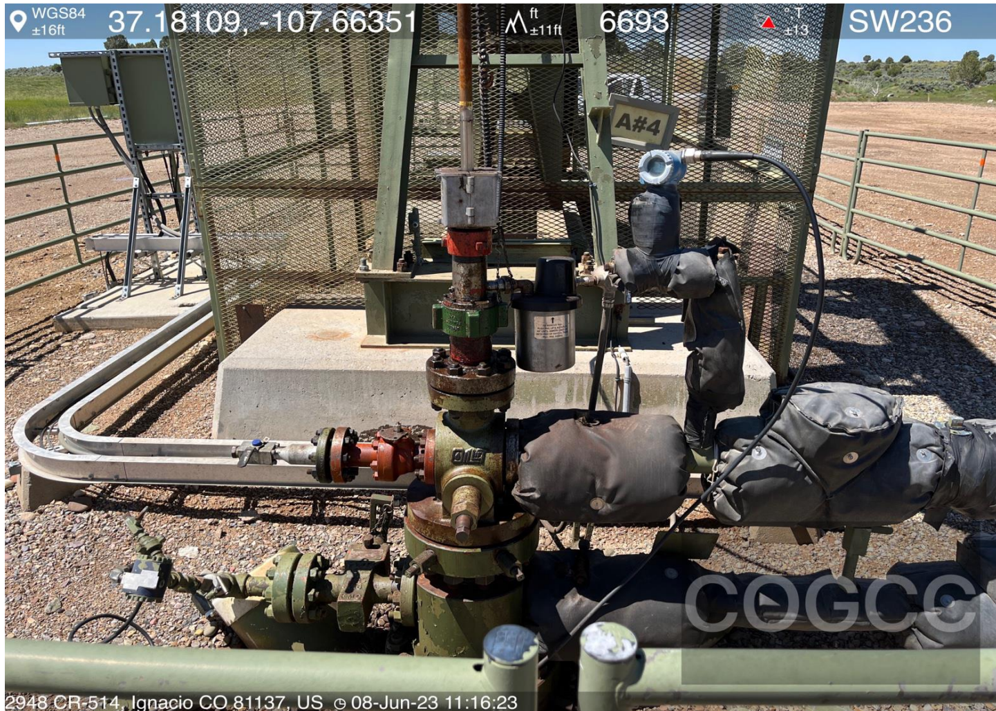
Photo #2. View of the A4 wellhead assembly.
