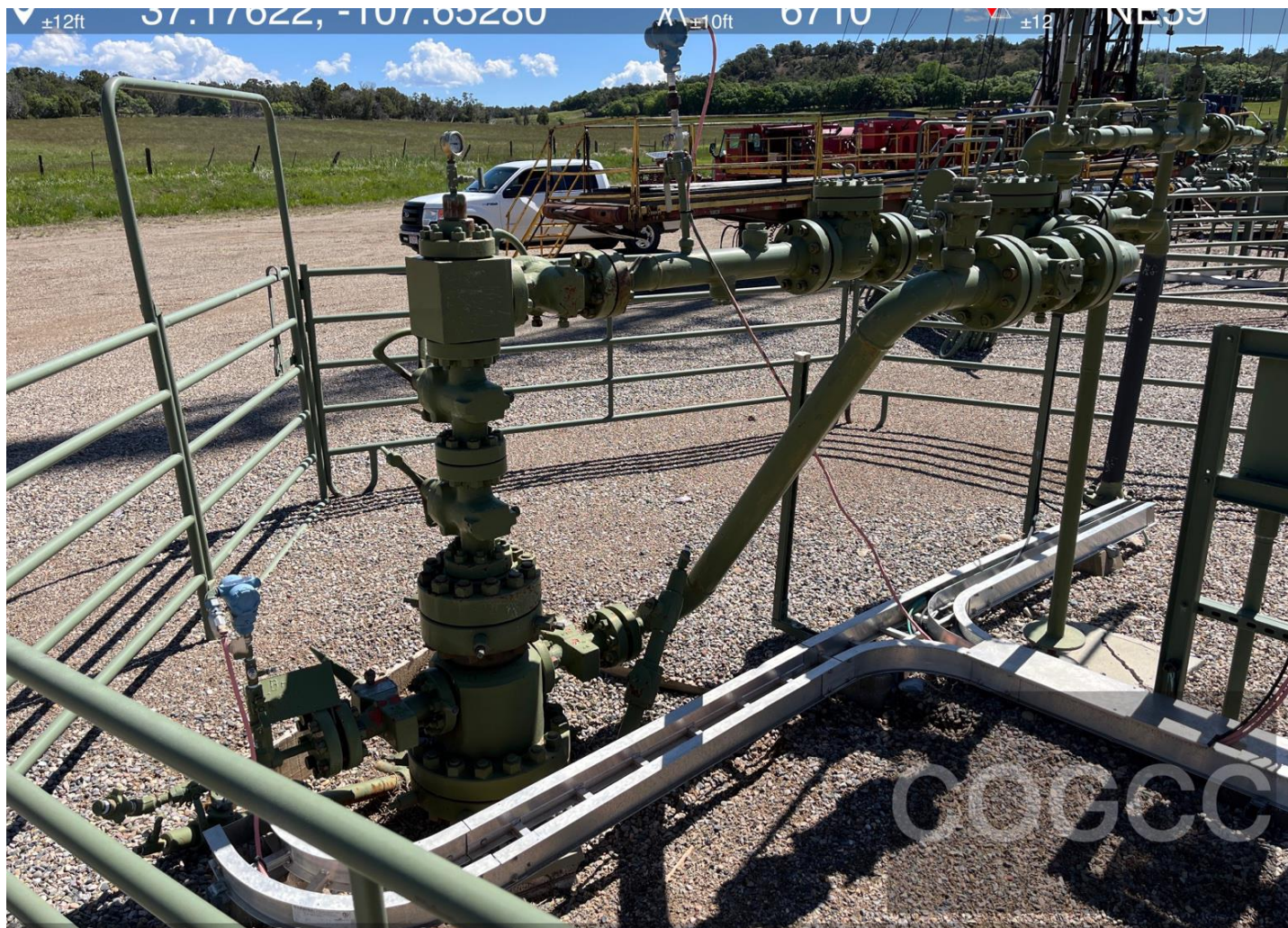
Photo #2. View of the A2 wellhead assembly.
