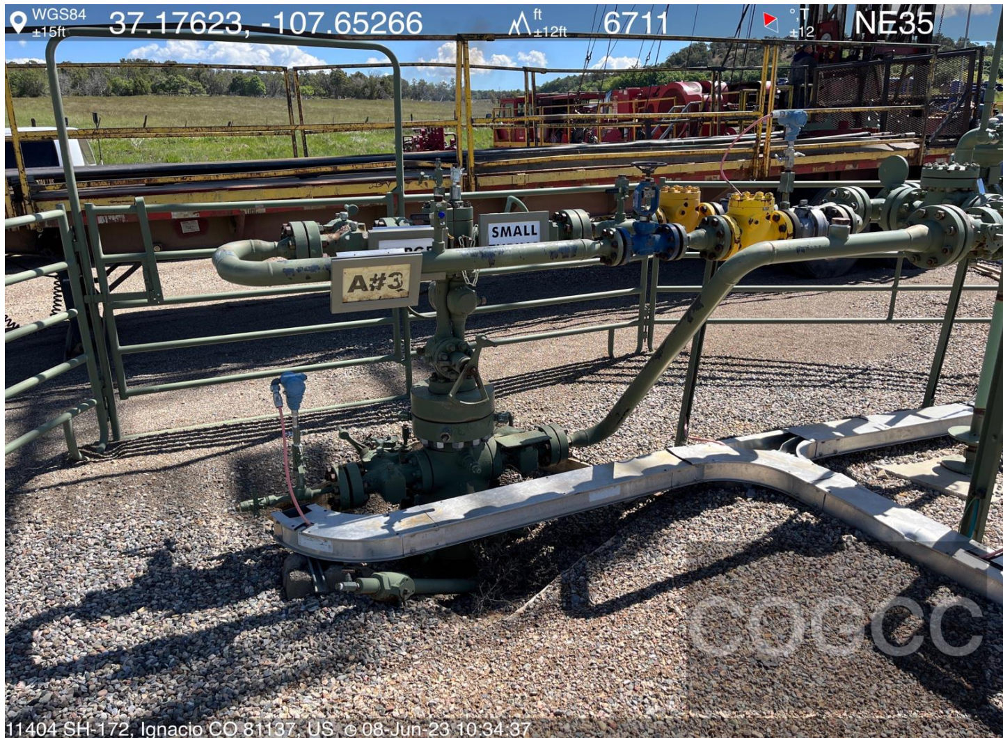
Photo #3. View of the A3 wellhead assembly.
