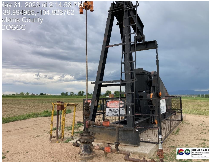
Pic 1 wellhead / pump jack
