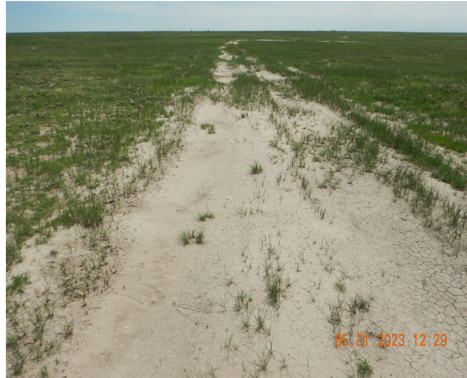
Photo 2. Photo taken along a central portion of the access road, facing South. See comments under Photo 1.
