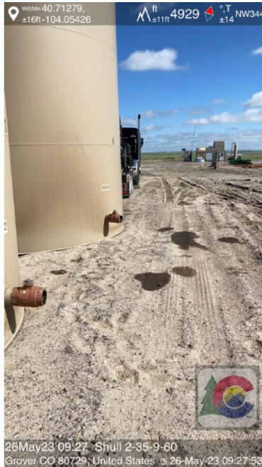
Photo 13 – Soil staining present & no OOSLAT on (2) 400-bbl crude oil ASTs
