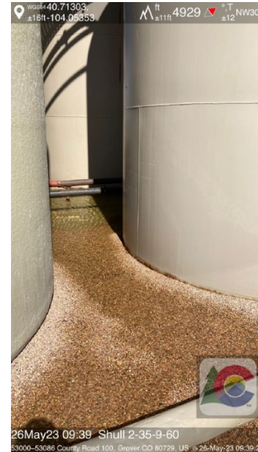
Photo 18 – Standing water in secondary containment for crude oil and produced water ASTs & corroded tank bottoms observed on all crude oil ASTs
