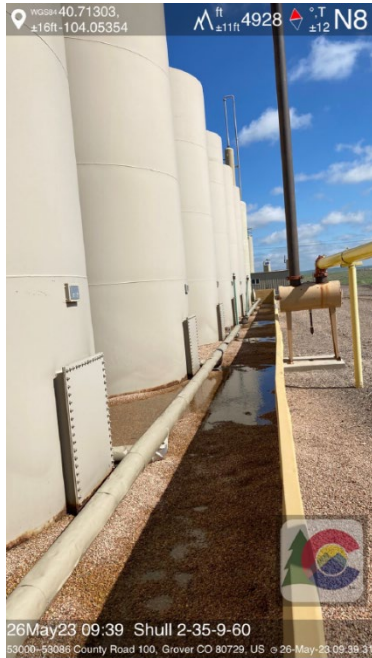
Photo 19 – Standing water in produced water & crude oil AST secondary containment
