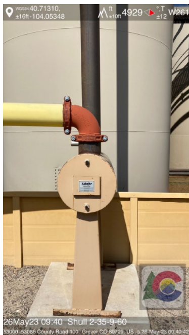
Photo 21 – Location of audible and olfactory leak (coupling on red elbow)
