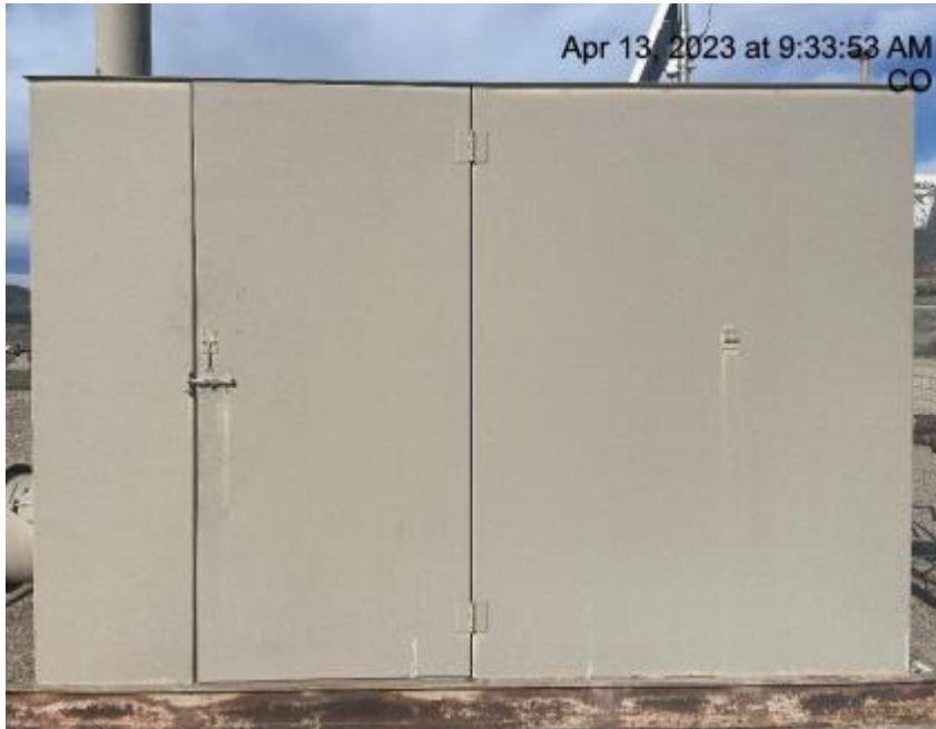
Photo # 5330 From Inspection 708900277 conducted on 04/13/2023 Meter calibration info not conspicuously posted
