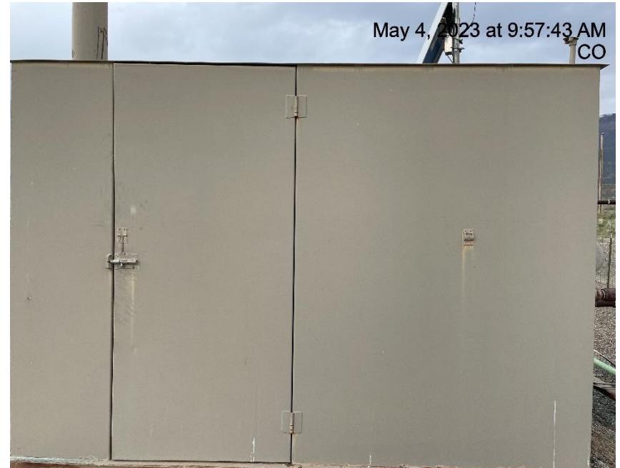
Photo # 6929 From Inspection 708900414 conducted on 05/04/2023 Meter calibration info not conspicuously posted
