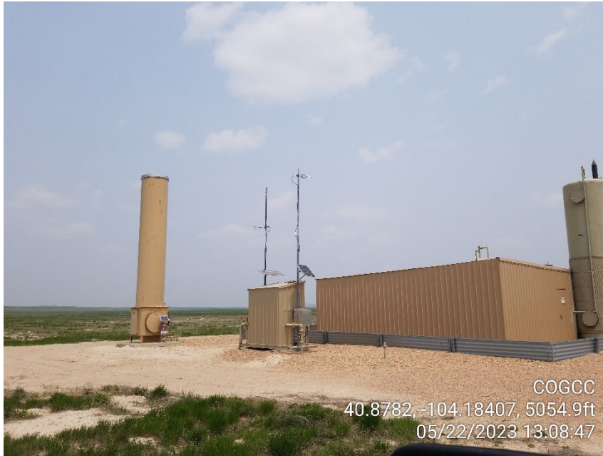
Photo 1 – ECD, Gas Meter and Heater Treater
