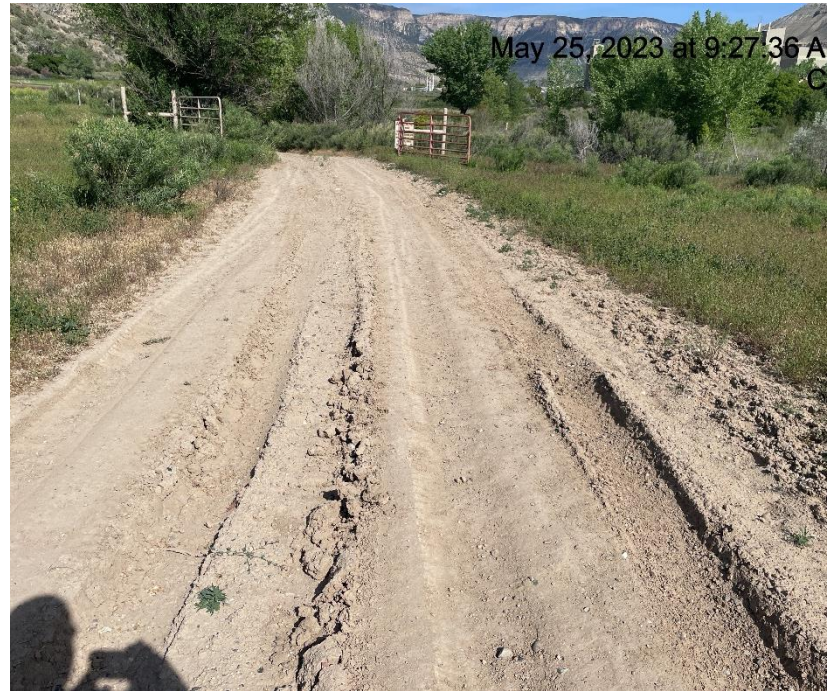
Photo # 8737 Lack of Stabilization/Compaction on spur road
