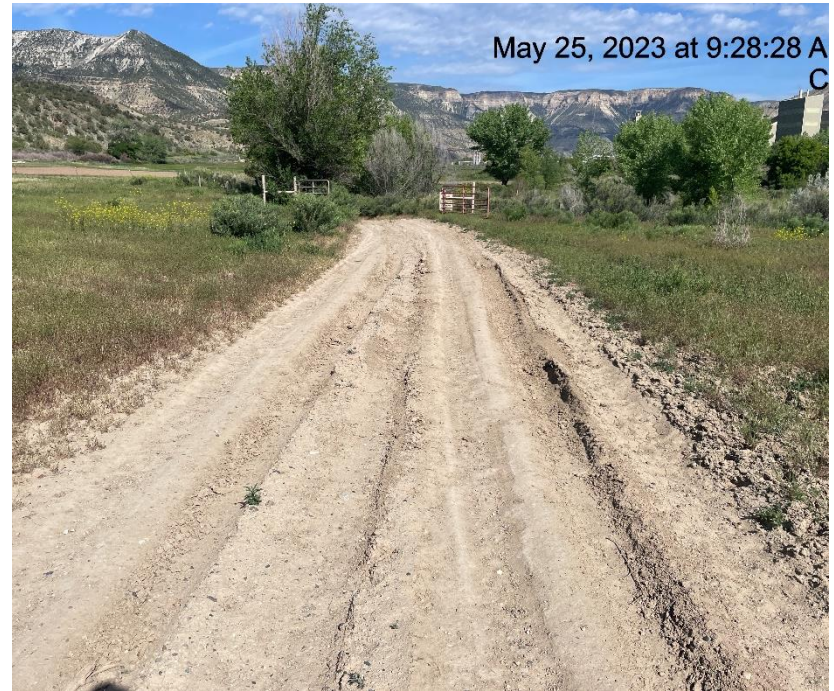
Photo # 8741 Lack of Stabilization/Compaction on spur road
