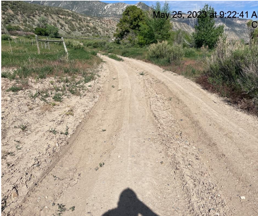
Photo # 8724 Lack of Stabilization/Compaction on location
