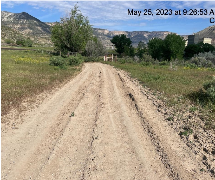
Photo # 8734 Lack of Stabilization/Compaction on spur road
