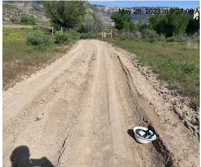
Photo # 8735 Lack of Stabilization/Compaction on spur road
