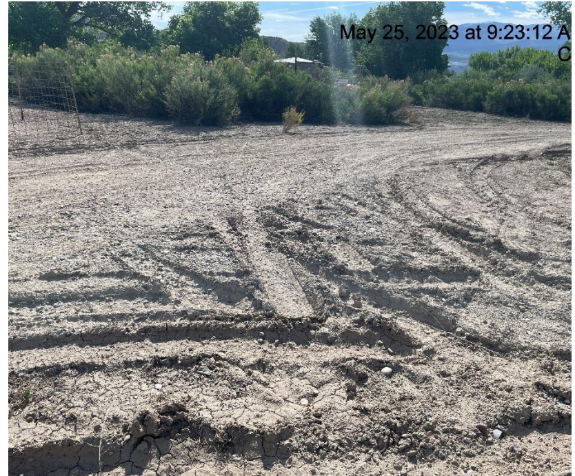
Photo # 8727 Lack of Stabilization/Compaction on location
