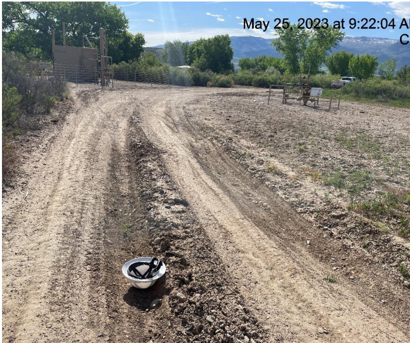
Photo # 8722 Lack of Stabilization/Compaction on location
