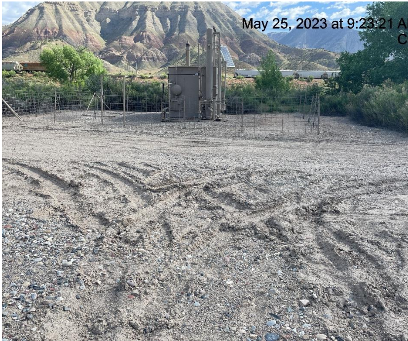
Photo # 8728 Lack of Stabilization/Compaction on location
