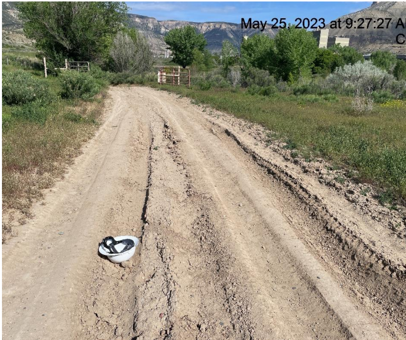
Photo # 8736 Lack of Stabilization/Compaction on spur road
