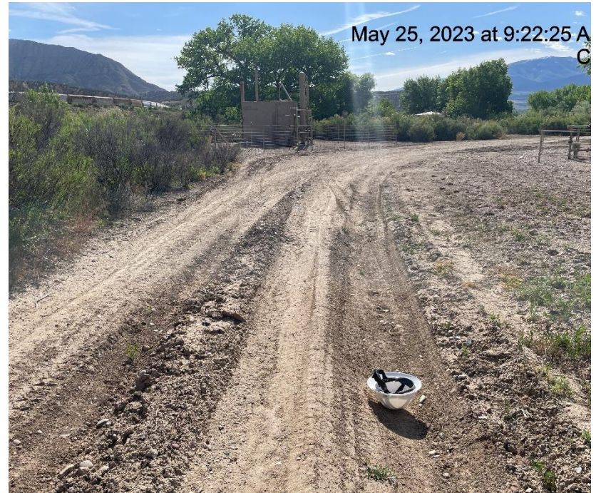
Photo # 8723 Lack of Stabilization/Compaction on location
