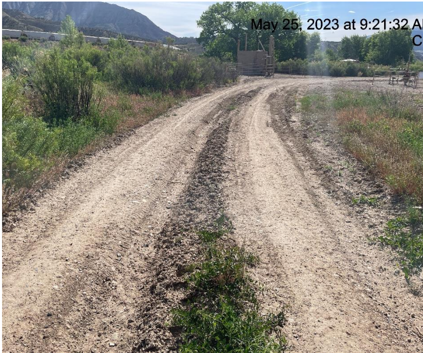
Photo # 8720 Lack of Stabilization/Compaction on location
