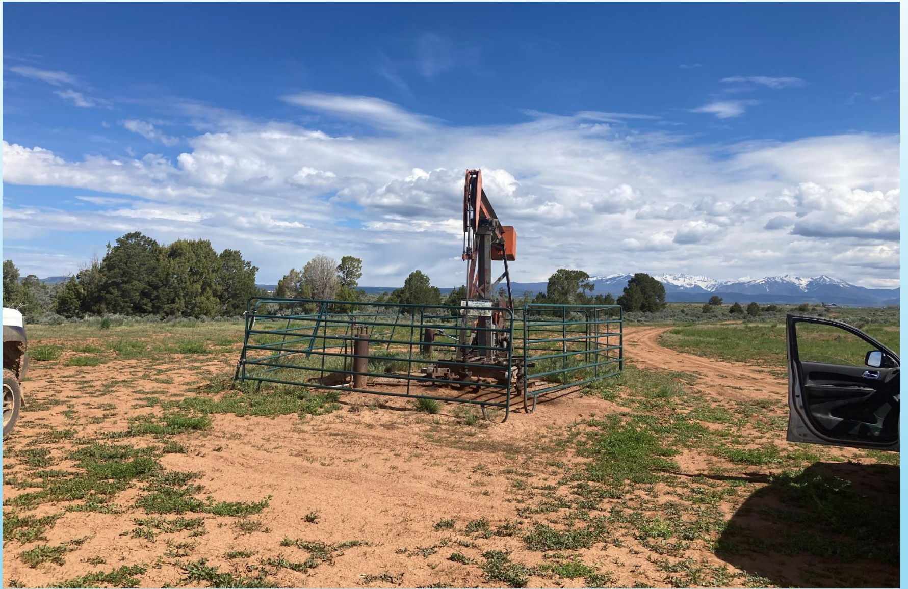
PHOTO 3: WELLHEAD AND EQUIPMENT
