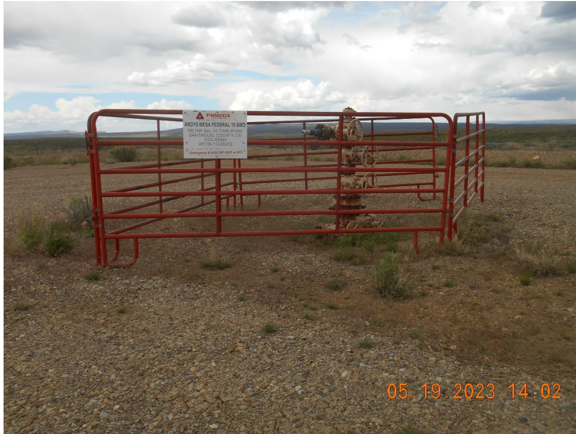
Injection Wellhead – Temporarily Abandoned
