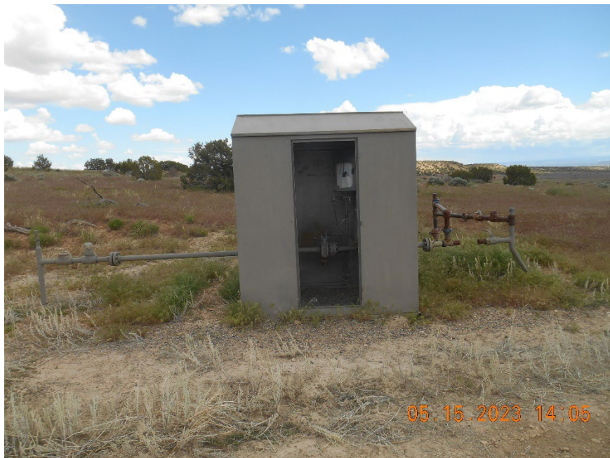
Meter housing and Compressor
