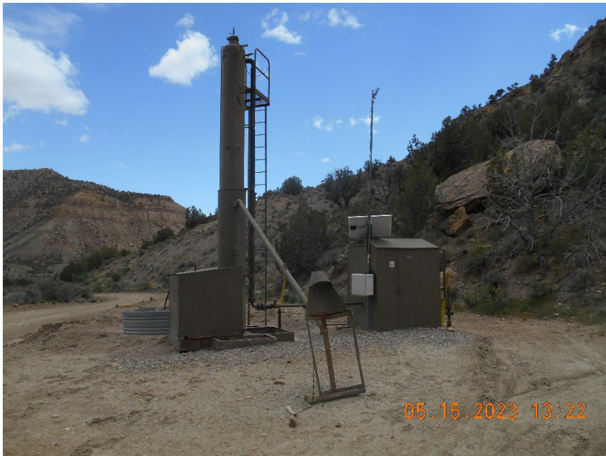
Meter housing, Dehydrator with blowdown tank
