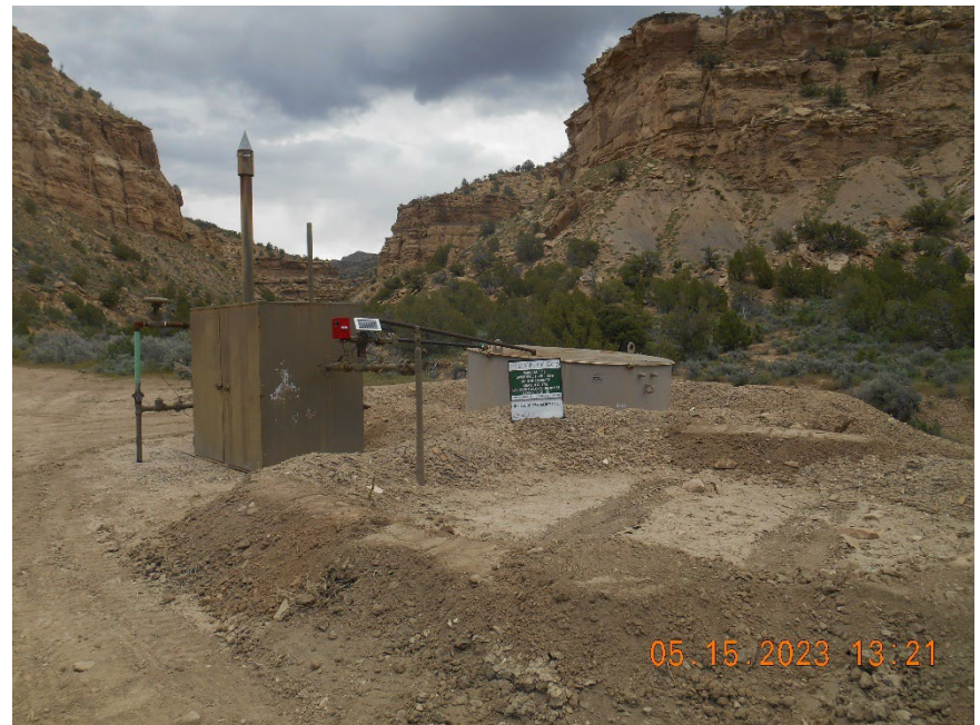
Separator with blowdown tank
