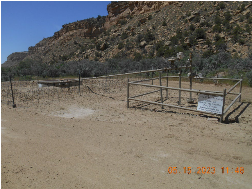
Wellhead with fence and sign.
