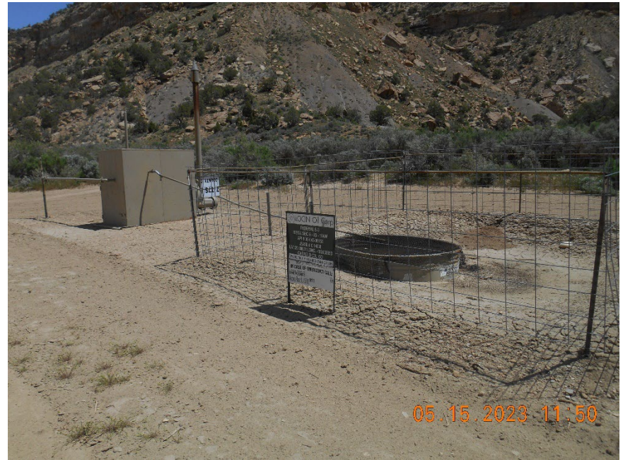
Separator with blowdown pit and fence
