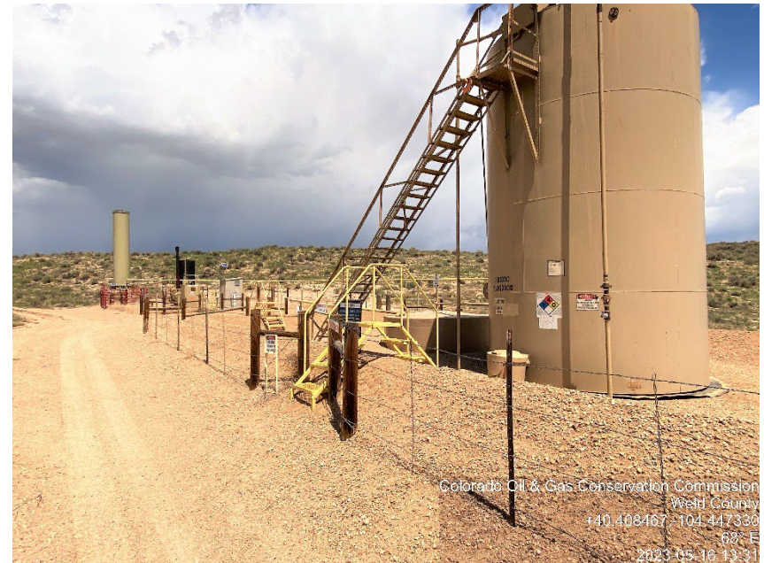
Photo #2 NHF 13-9, 24-9 Battery site Inactive | Shut-down Equipment documented: Loc. # 331573
