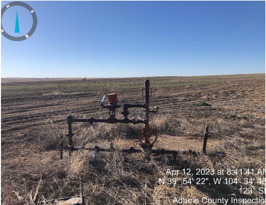
Photo# 3 Well Head.
