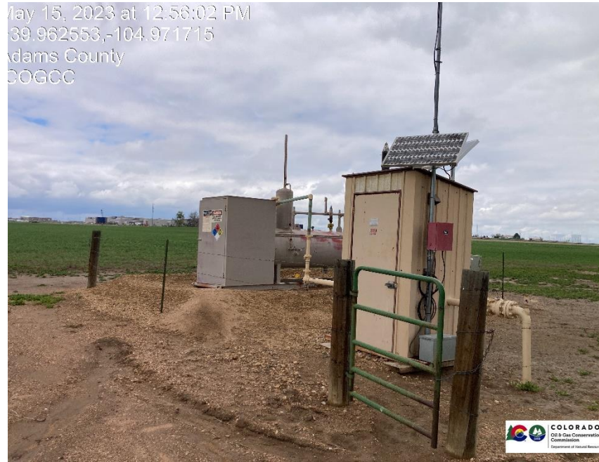
Pic 3 Separator, GMR
