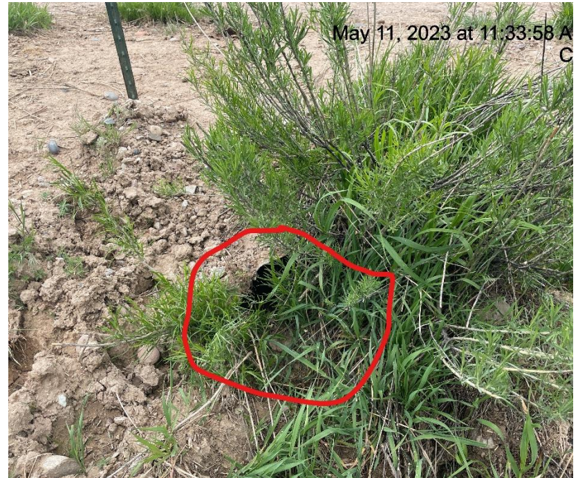
Photo # 7568 Culvert needs maintenance (unable to locate other end of culvert, possibly crimped & buried under sediment)
