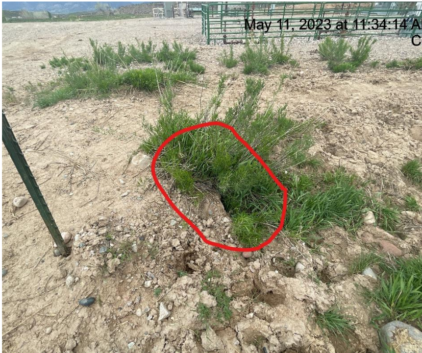
Photo # 7569 Culvert needs maintenance (unable to locate other end of culvert, possibly crimped & buried under sediment)
