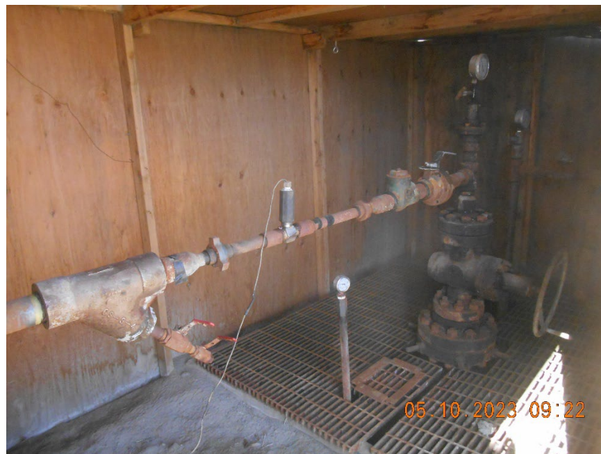
Wellhead inside housing
