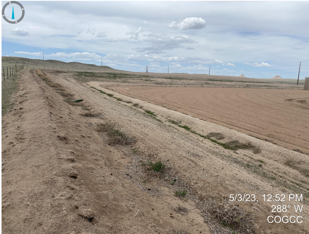
Photo 14. Cut slopes and perimeter stormwater controls will need to be properly stabilized and undesirable vegetation will need to be managed during the next growing season.
