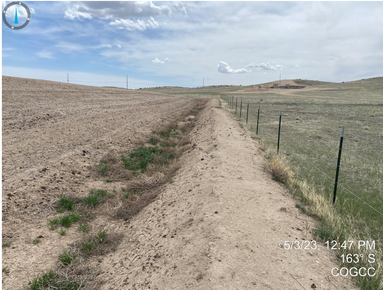
Photo 11. Topsoil stockpile void of any protections and/or vegetation and undesirable plant species observed in the stormwater ditch.
