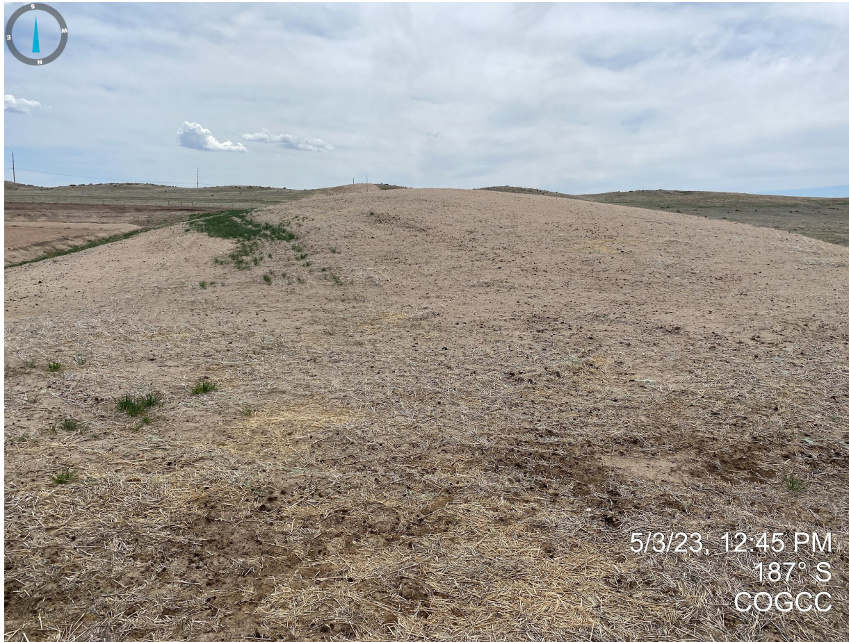
Photo 8. Topsoil stockpile does not appear to be properly stabilized per Rule 1002.c. Additional BMPs will need to be implemented to stabilize the topsoil.
