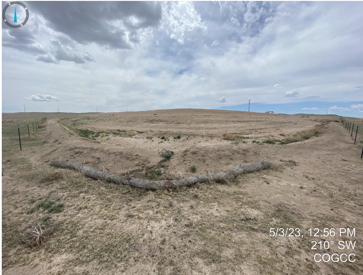
Photo 19. Cut slopes and stormwater BMPs will need to be properly stabilized to protect against wind and water erosion. Degraded straw wattles do not appear adequate and will require maintenance, repairs, or replacements.
